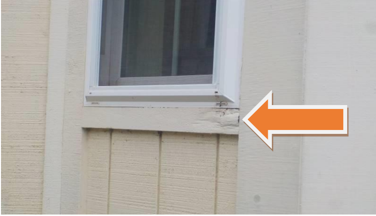
Item #26-Exterior trim-At the rear of the home, wood damage to the 1x4 window trim
