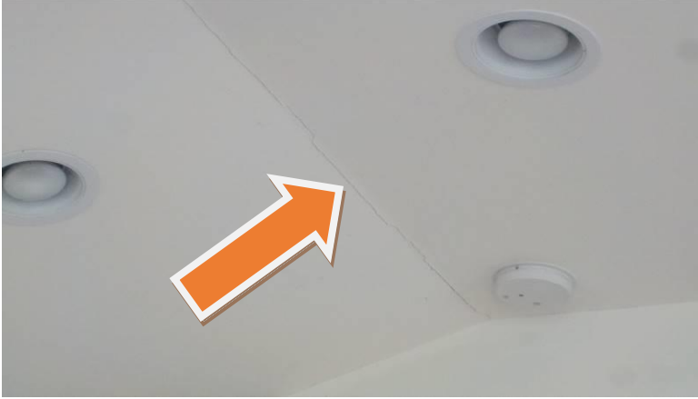
Item #219-Hallway, door-At the door to the closet, there is a hole in the hallway side of the door
