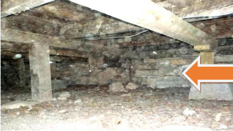
Item #117-Crawl space, foundation-Along the north side of the home (front), concrete rubble has been used as a foundation
