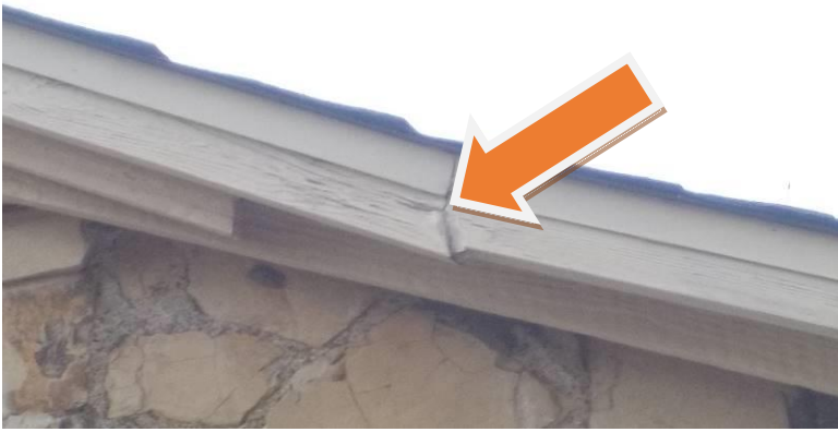
Item #19-Rain gutters-At the rear of the home, the gutters are blocked with debris, mainly at the gutter to downspout connection
