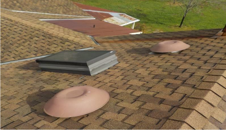
Note-Roof-The composite shingle roofing material all appears to be in good condition/below; over the great room
