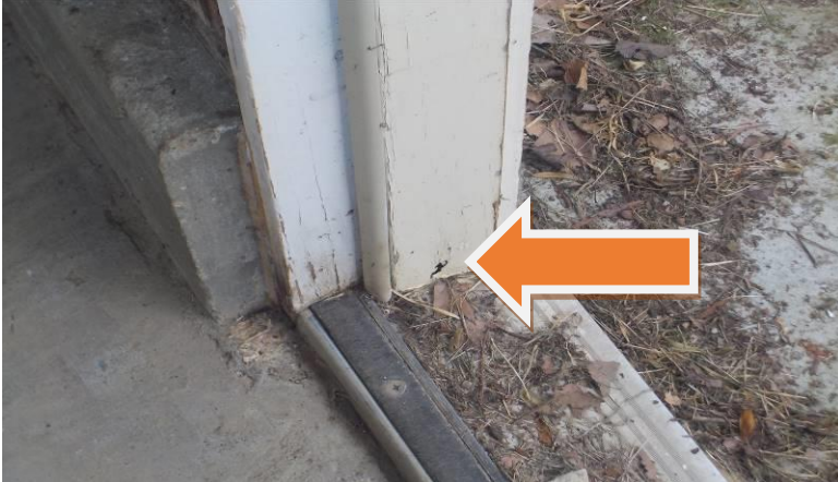
Item #67-Kitchen, drainage-This gray ribbed drain line should be re-routed to be higher than the bottom of the sink/see 3-photos below
