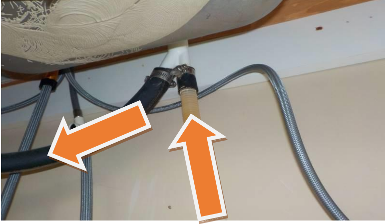
Item #88-Water heater-Seismic straps are required 1/3 down from the top and 1/3 up from the bottom of the heater tank
