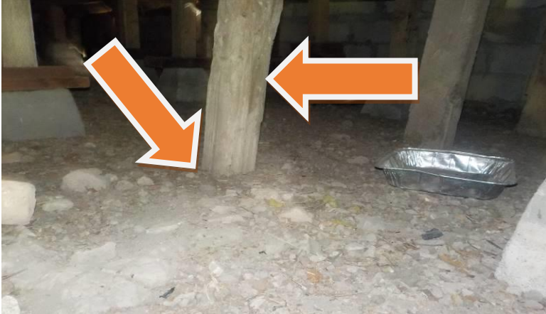
Item #'s 113/118-Crawl space, columns/girders-Many of the columns are not on piers, but buried in the soil and have wood damage
