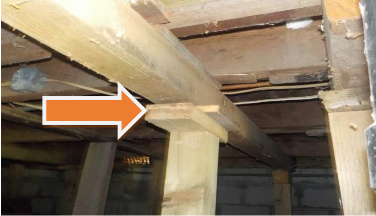
Item #'s 113/118-Crawl space, columns/girders-The columns have spacers between the top of the columns and the girders/piers/not secured
