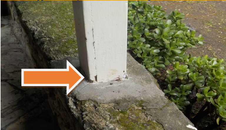
Item #25-Supports-Mainly at the west end of the porch/veranda, there is some wood damage to the 4x4 support posts, various posts
