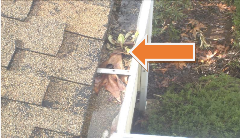
Item #19-Rain gutters-At the rear of the home, the gutters are blocked with debris, mainly at the gutter to downspout connection
