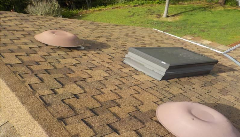
Note-Roof-The composite shingle roofing material all appears to be in good condition/below; over the great room
