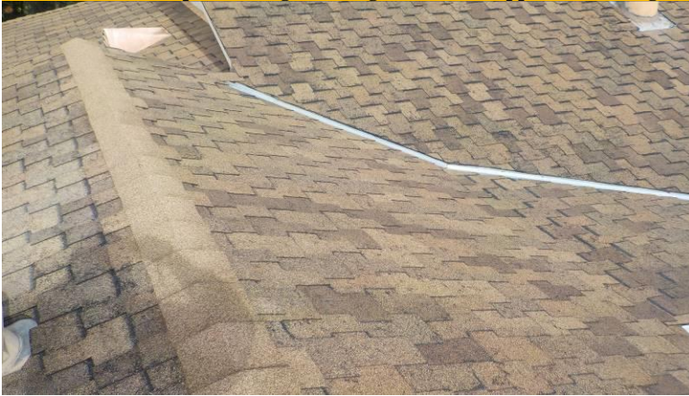
Note-Roof-The composite shingle roofing material all appears to be in good condition/below; over the laundry room and living room
