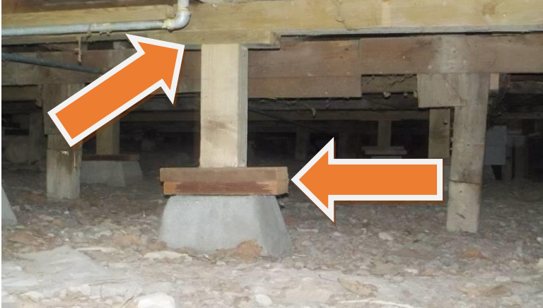
Item #'s 113/118-Crawl space, columns/girders-Many of the columns have spacers between the top of the columns and the girders/not secured
