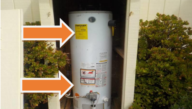
Item #88-Water heater-The water temperature in the home is at 136.9 degrees (too hot) / 115-120 degrees is recommended
