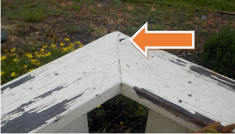
Item #13-Deck-At the rear deck, wood damage to the bottom rail framing
