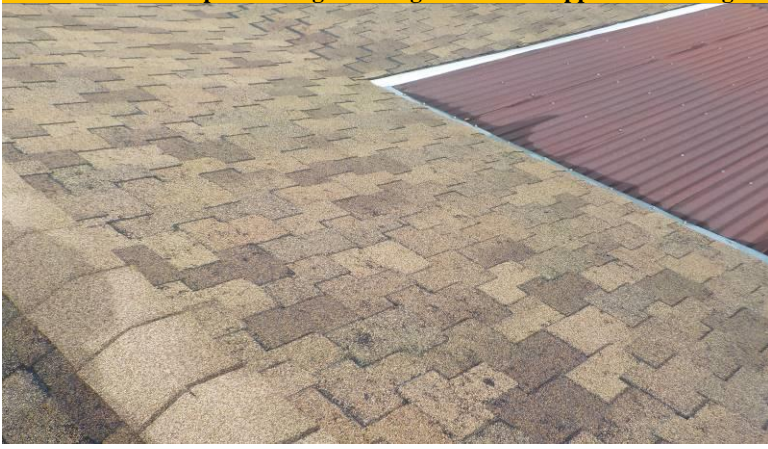
Note-Roof-The composite shingle roofing material all appears to be in good condition/below; over the laundry room
