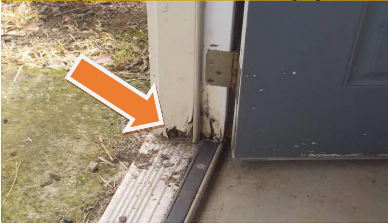
Item #59-Garage, exterior trim-On the north side of the garage, there is wood damage to the door frame and trim down near the threshold
