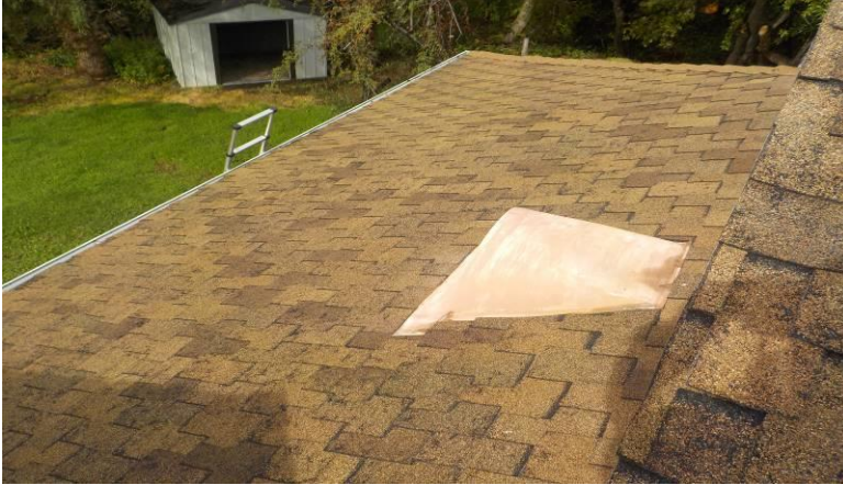
Note-Roof-The composite shingle roofing material all appears to be in good condition/below; over the primary bedroom and kitchen area
