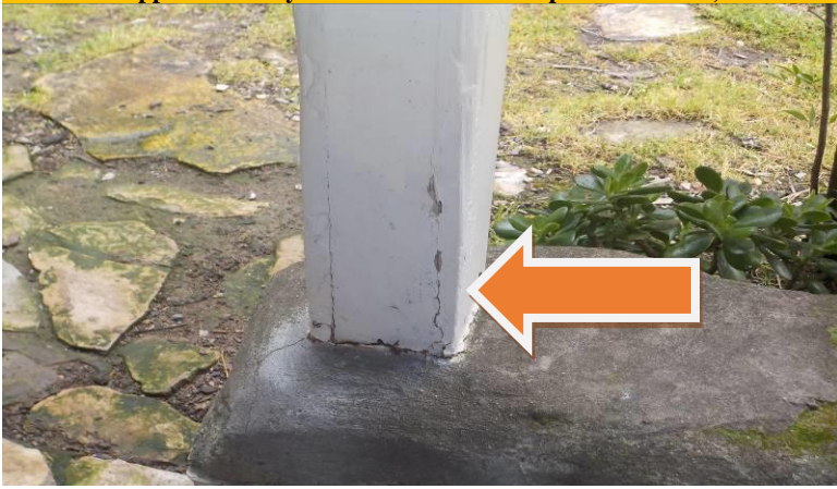
Item #25-Supports-Mainly at the west end of the porch/veranda, there is some wood damage to the 4x4 support posts, various posts
