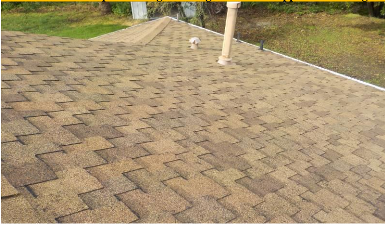
Note-Roof-The composite shingle roofing material all appears to be in good condition/below; over the primary bedroom
