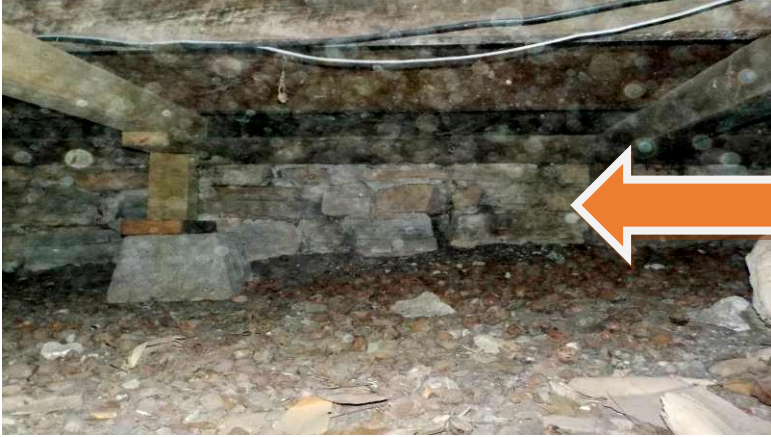
Item #117-Crawl space, foundation-Along the north side of the home (front), concrete rubble has been used as a foundation
