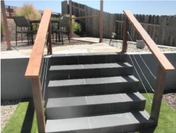
Nongraspable handrails at the backyard upper patio steps.
