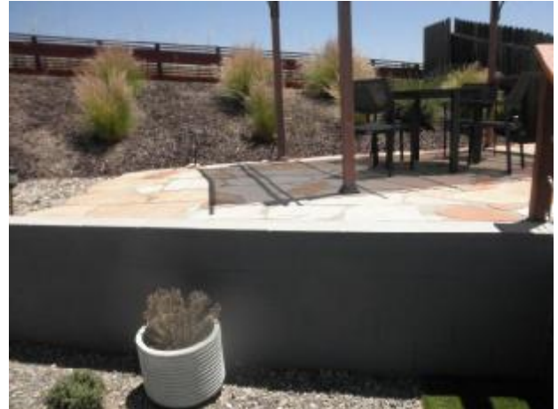
No railing installed at the backyard upper patio.
