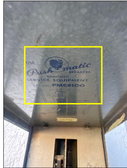
The service panel brand was Pushmatic.
