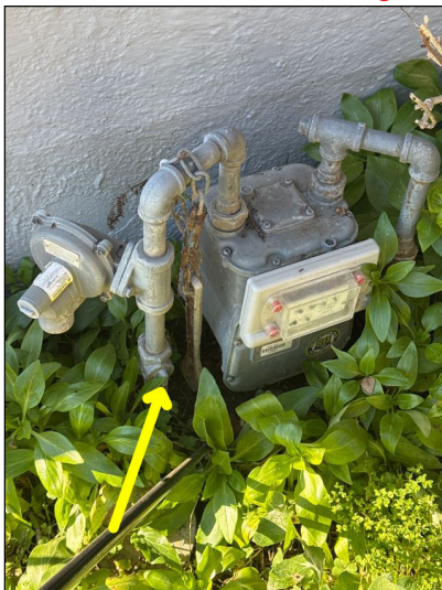
Main gas shut off to the home.
