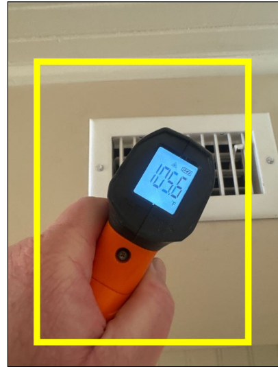
The supply air temperature at the registers should be 100 °F - 125 °F + to be considered running efficiently.
