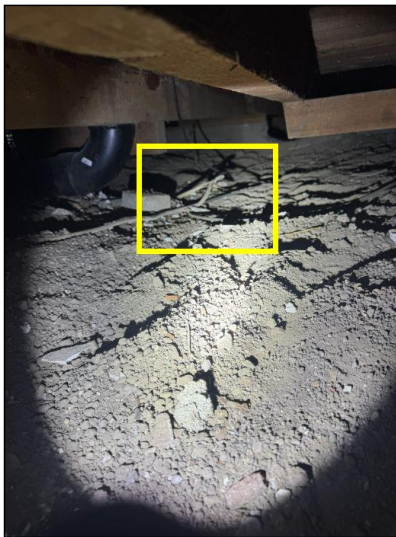
Electrical wires visible in the crawlspace had splices exposed to touch.
