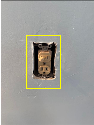
At the time of the inspection, an electrical receptacle cover plate was missing
