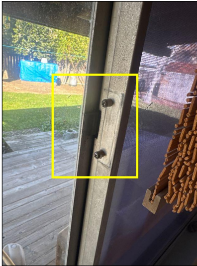
A window had inoperable hardware (broken lock).
