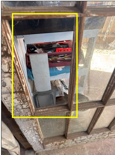
broken glass in door
