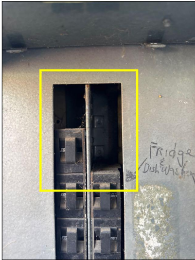
Filler plates missing in open breaker slot in the dead front cover of the service panel
