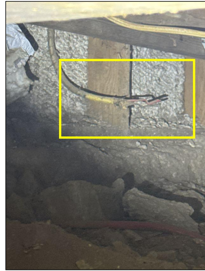
Electrical wires visible in the crawlspace terminated outside of the junction box.
