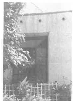
Despite their utility, garden-box windows such as this did not exist during this home's Period of Significance.
