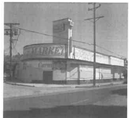
Doors and windows have been removed from this building (in favor of a rear-facing parking lot), to the detriment of the street.
