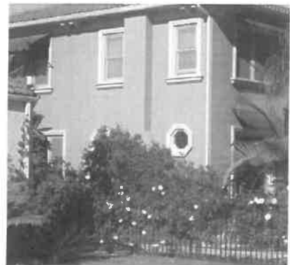
Foam plant-ons and pre-cast concrete are materials that would not have been originally used on this historic house.
