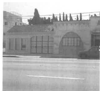
Concrete block is not a material that is original to this Spanish Colonial building.
