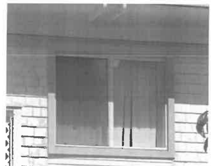
An inappropriately sized aluminum window diminishes the historic value of a house.
