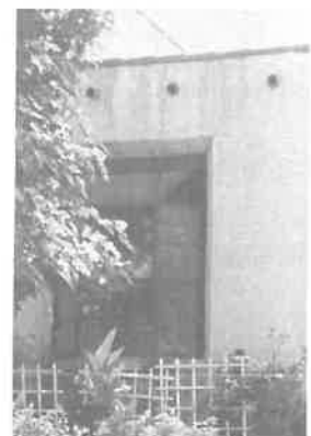
Despite their utility, garden-box windows such as this did not exist during this home's Period of Significance.
