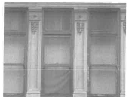
These windows should be repaired rather than replaced.
