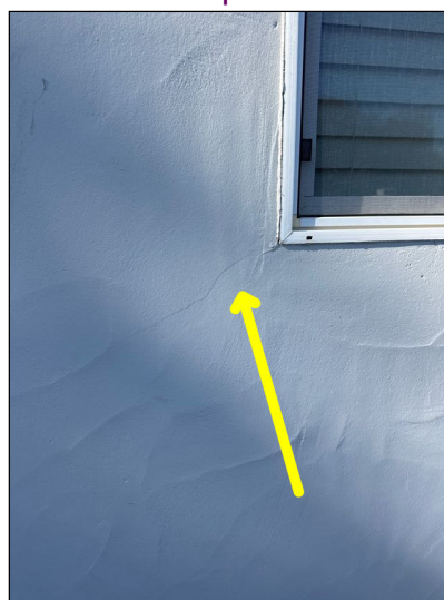
Monitor: Normal cracking was visible in stucco covering exterior walls of the home at the time of the inspection.
