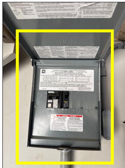
Sub panel to the pool/spa
