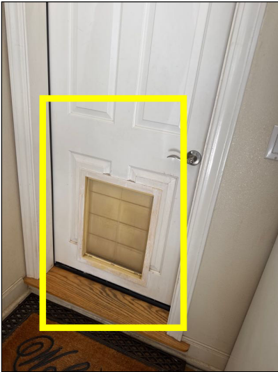
Pet doors in firewall doors are a breach in the firewall.
