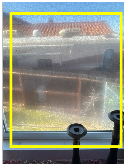
Staining and etching of the glass at the window indicated a loss of thermal integrity.
