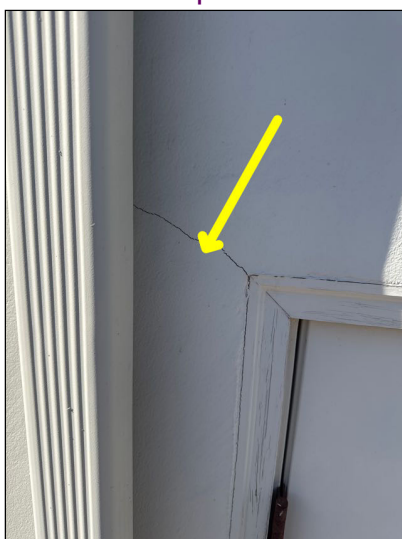
Monitor: Normal cracking was visible in stucco covering exterior walls of the home at the time of the inspection.
