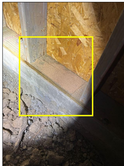
Termite dropping visible in the crawlspace walls indicated infestation by wood-destroying insects.
