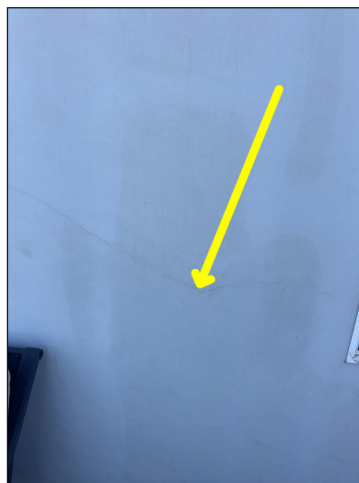
Monitor: Normal cracking was visible in stucco covering exterior walls of the home at the time of the inspection.
