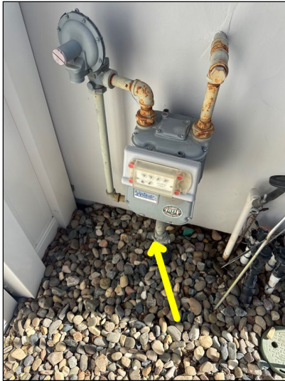
Main gas shut off to the home.
