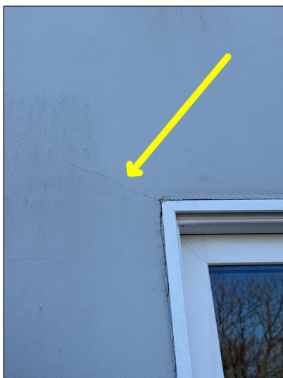
Monitor: Normal cracking was visible in stucco covering exterior walls of the home at the time of the inspection.
