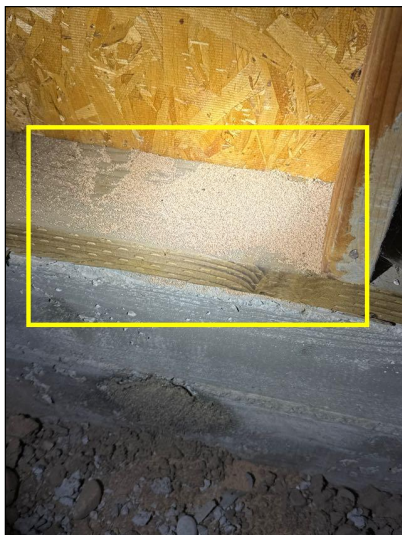
Termite dropping visible in the crawlspace walls indicated infestation by wood-destroying insects.
