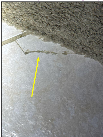
The Hallway had cracked floor tiles visible at the time of the inspection.
