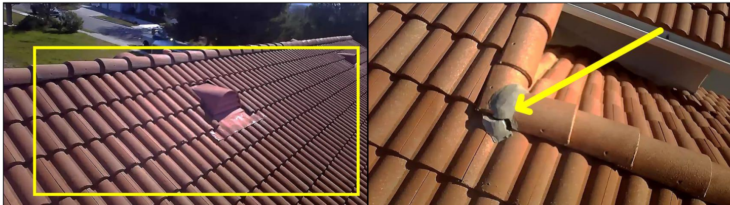
Roof ridge cap tiles are mortar sealed at intersections, the mortar is cracked
