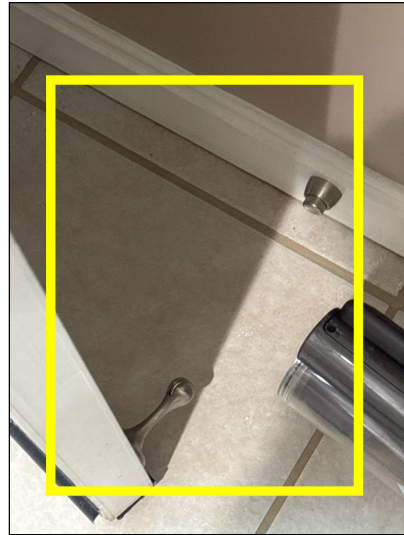
Door stops that prevent the door from self-closing are considered a breach in the firewall.
