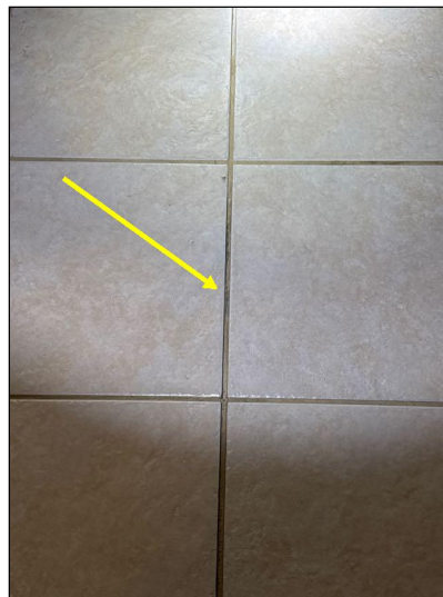
Grout lines in the tile floor of the Hallway needed maintenance at the time of the inspection.
