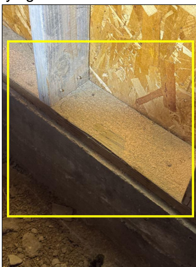
Termite dropping visible in the crawlspace walls indicated infestation by wood-destroying insects.
