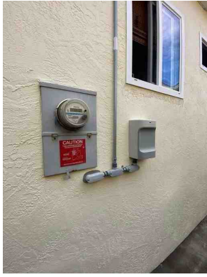
Electric Panel Service
