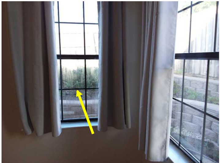
A window(s) may have a broken hermetic seal which you may wish to have replaced. This is evident from fogging, or condensation forming between the panes of glass that confirm that the seal has failed.
