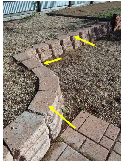
Some of the planter block-caps are loose or missing and should be serviced.
