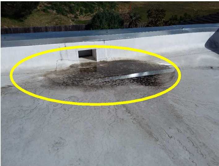
There are areas of the roof that are sunken or bellied and is holding water which should be evaluated and serviced by a licensed roofing contractor.
