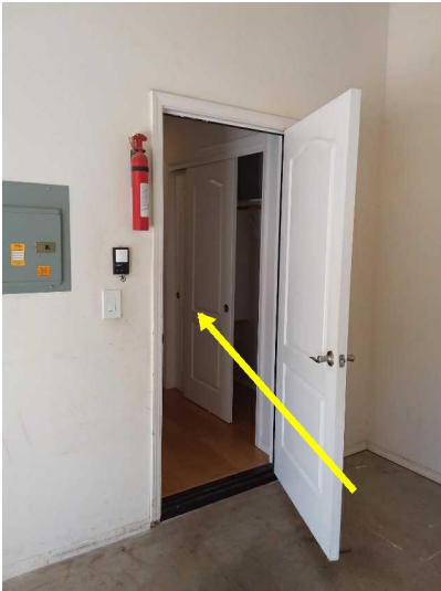
The house entry door is not a fire rated, self-closing and latching door, which should be serviced.
