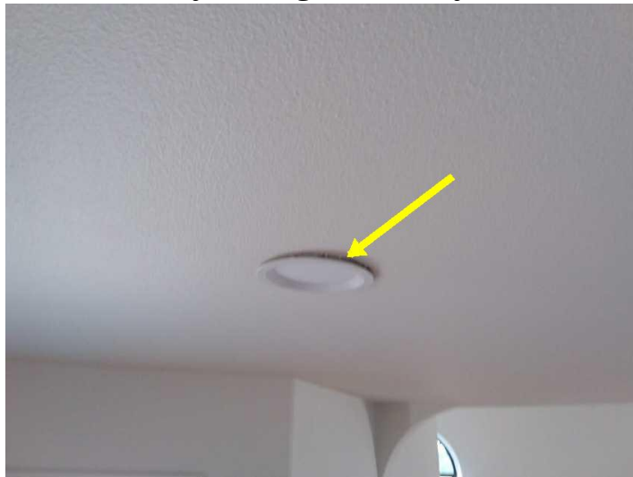
A ceiling light is not fully secure which should be serviced.
