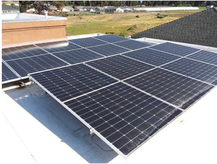
9 panels on roof
