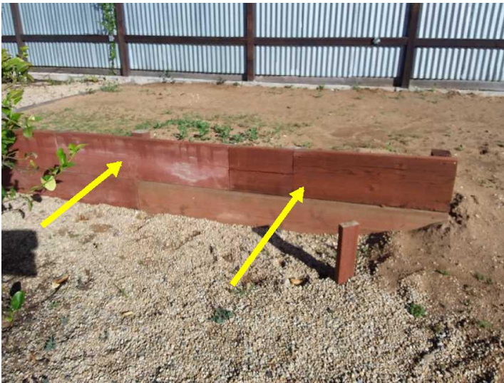
The wooden planks at the rear of the property have no structural value, and are intended to inhibit surface soil movement, and should be periodically monitored for damage or stability.
