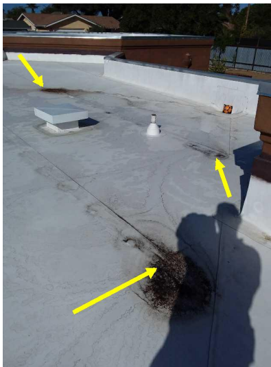
There are areas of the roof that are sunken or bellied and is holding water which should be evaluated and serviced by a licensed roofing contractor.
