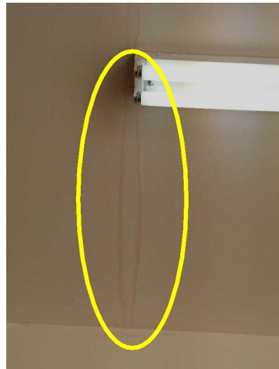
There is a moisture stain on the garage ceiling, the cause of which should be explained or explored further. However, we not unable to confirm that is being caused by an active leak.
