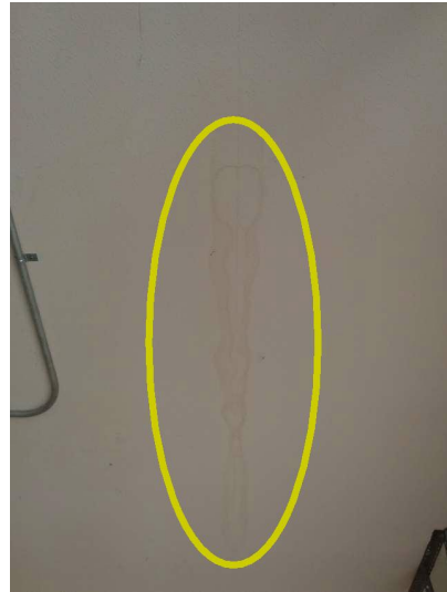
There is a moisture stain on the garage ceiling, the cause of which should be explained or explored further. However, we not unable to confirm that is being caused by an active leak.
