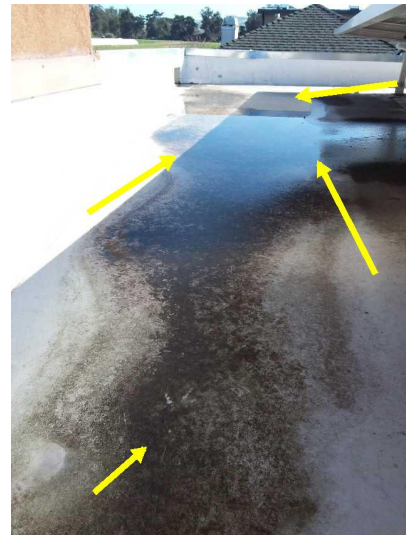
There are areas of the roof that are sunken or bellied and is holding water which should be evaluated and serviced by a licensed roofing contractor.
