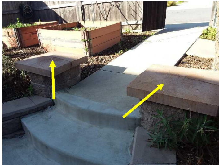
Some of the planter block-caps are loose or missing and should be serviced.
