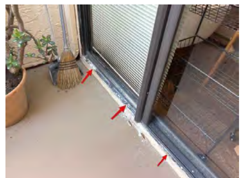
North Office, metal door jamb corroded
