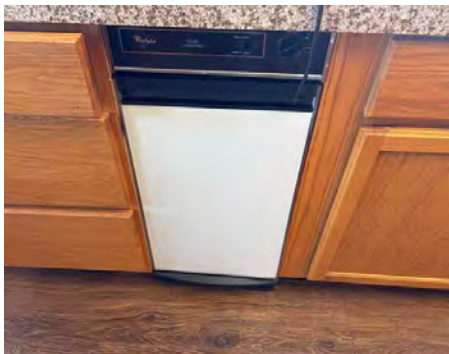
Trash Compactor Operable
