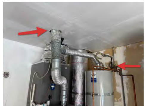
Airs gaps between flue pipe, water pipes and ceilings/walls.
