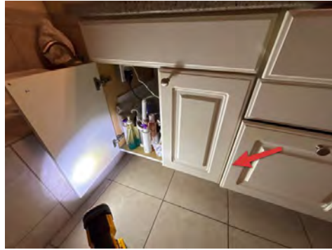
Primary Bathroom, left hand sink cabinet, loose hinge
