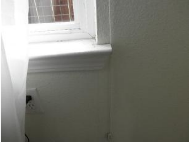
Evidence of a leak at the single hung window in the master bedroom.
