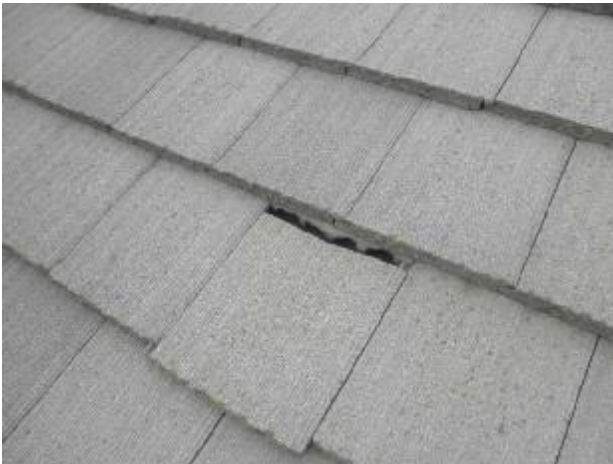
Cracked and displaced tiles on the north facing slope.
