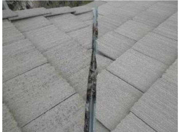
The leaves and debris need to be cleared out of the valleys.
