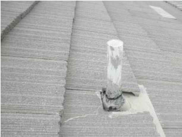
Deteriorated sealant at the vent flashings.
