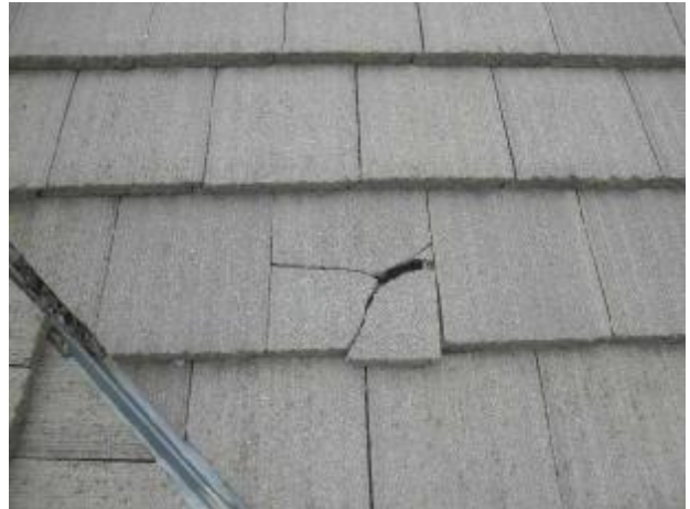
Broken tile on the east facing slope.
