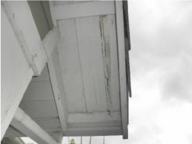
Evidence of a leak with moisture damage to the eave.
