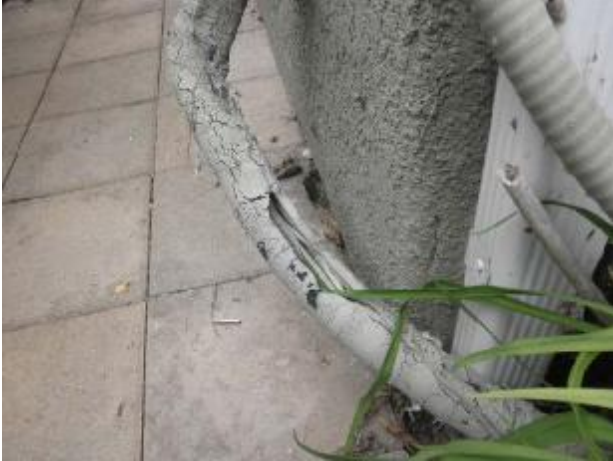
Deteriorated insulation at the A/C low-pressure refrigerant line.
