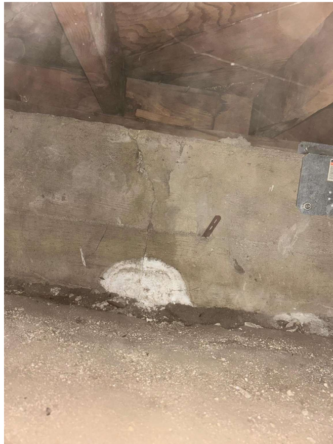
Crack in foundation
