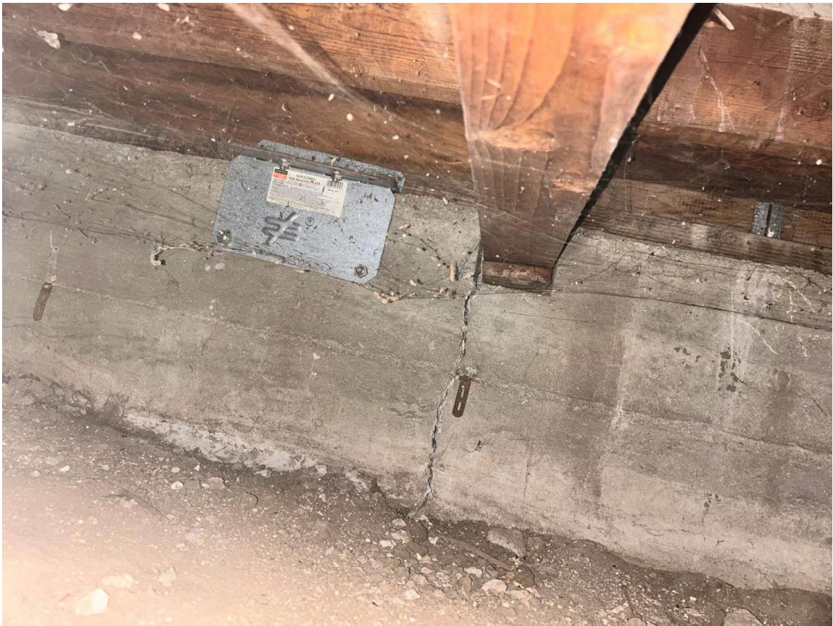
Crack in foundation
