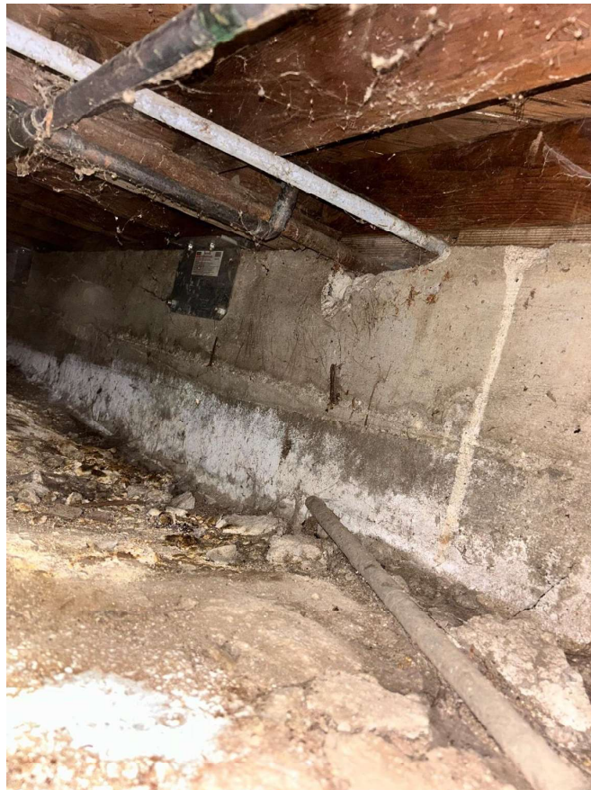
Wet soil along rear wall
