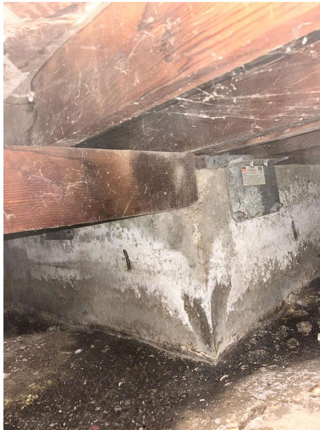
Wet soil along rear foundation wall
