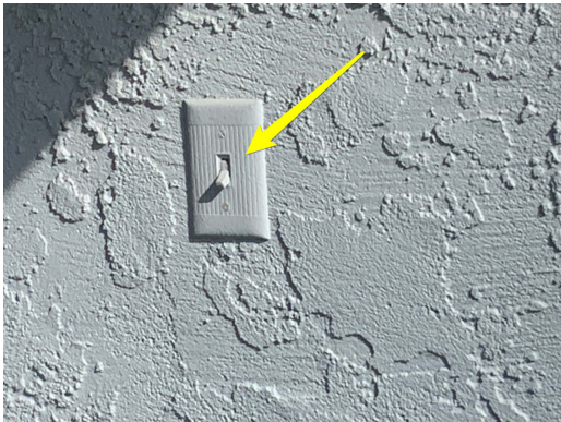
Switch needs a proper weather tight cover
