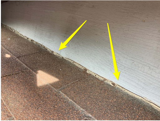
No exposed metal flashing
