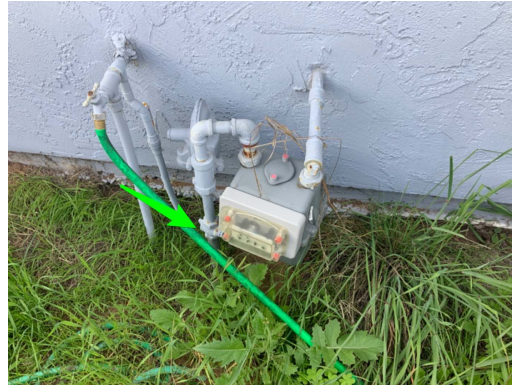
Main gas shut off valve
