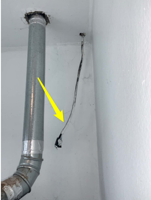
In the laundry room above the water heater
