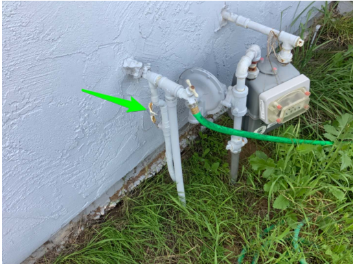
Main water shut off valve
