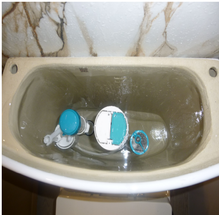
TOILET IN HALL BATHROOM RUNS CONSTANTLY RECOMMENDS REPLACING FLOATER IN TANK
