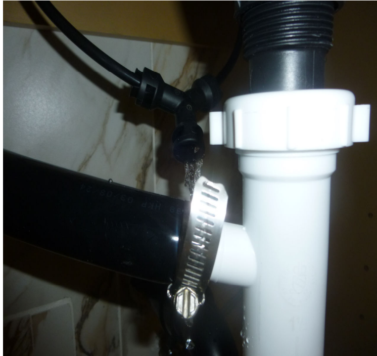
HOT AND COLD WATER SUPPLY LINES UNDER HALL BATHROOM LEAKS REPAIR NEEDED RECOMMEND FURTHER EVALUATION
