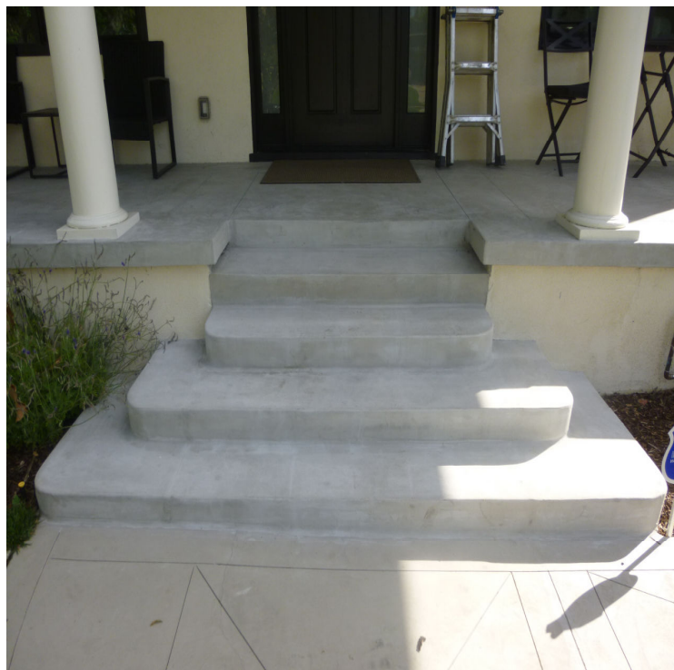
SEVERAL EXTERIOR STEPS FRONT OF HOUSE MISSING AT LEAST ONE HANDRAIL INSTALLMENT NEEDED
