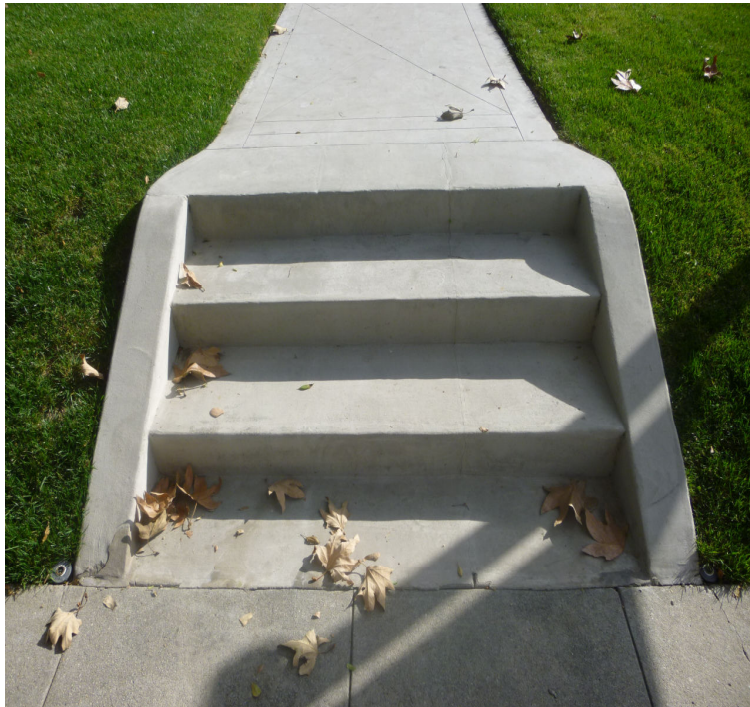
SEVERAL EXTERIOR STEPS FRONT OF HOUSE MISSING AT LEAST ONE HANDRAIL INSTALLMENT NEEDED
