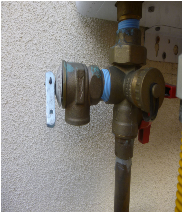
MISSING T.P.R PIPE ON WATER HEATER PIPE NEEDS TO BE COPPER ARE GALVANIZED INSTALLMENT NEEDED
