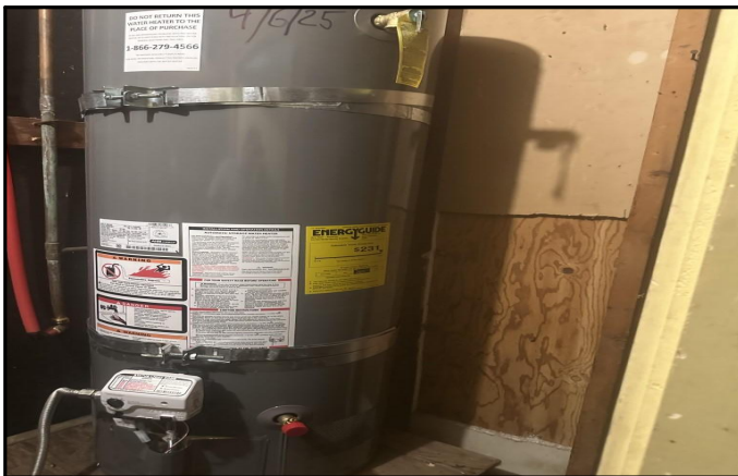
STRAPPED WATER HEATER
