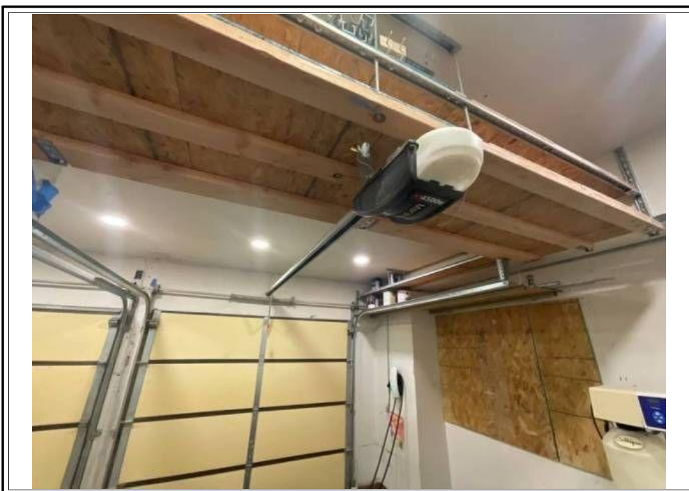
GARAGE AUTOMATIC GARAGE DOOR OPENER
