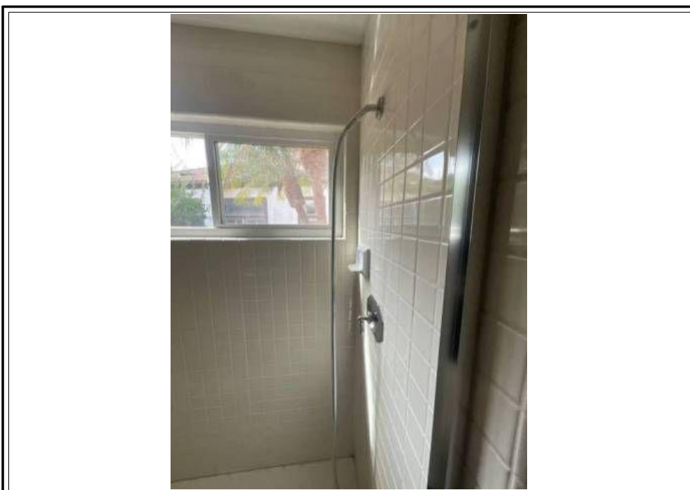
BATHROOM 1 BATHROOM SHOWER HEAD
