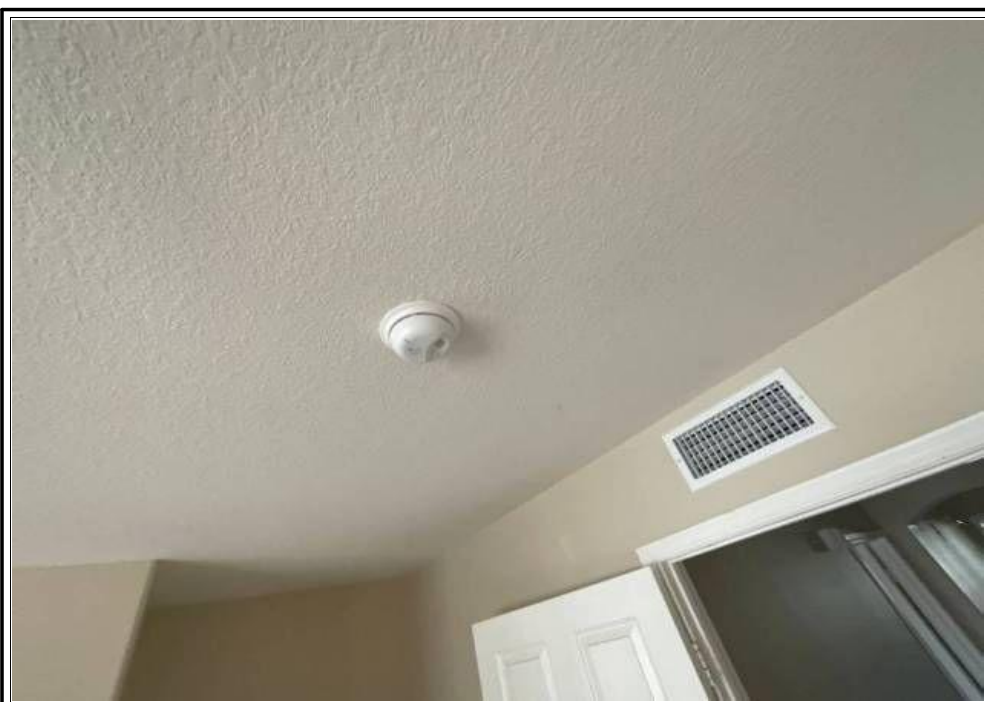
BEDROOM 2 SMOKE DETECTOR
