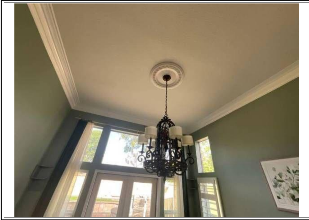
DINING ROOM LIGHT FIXTURES
