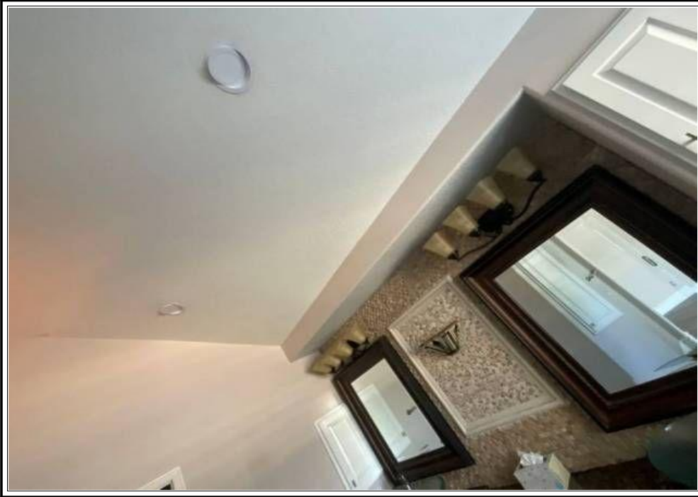
BATHROOM 3 TRACK LIGHTING
