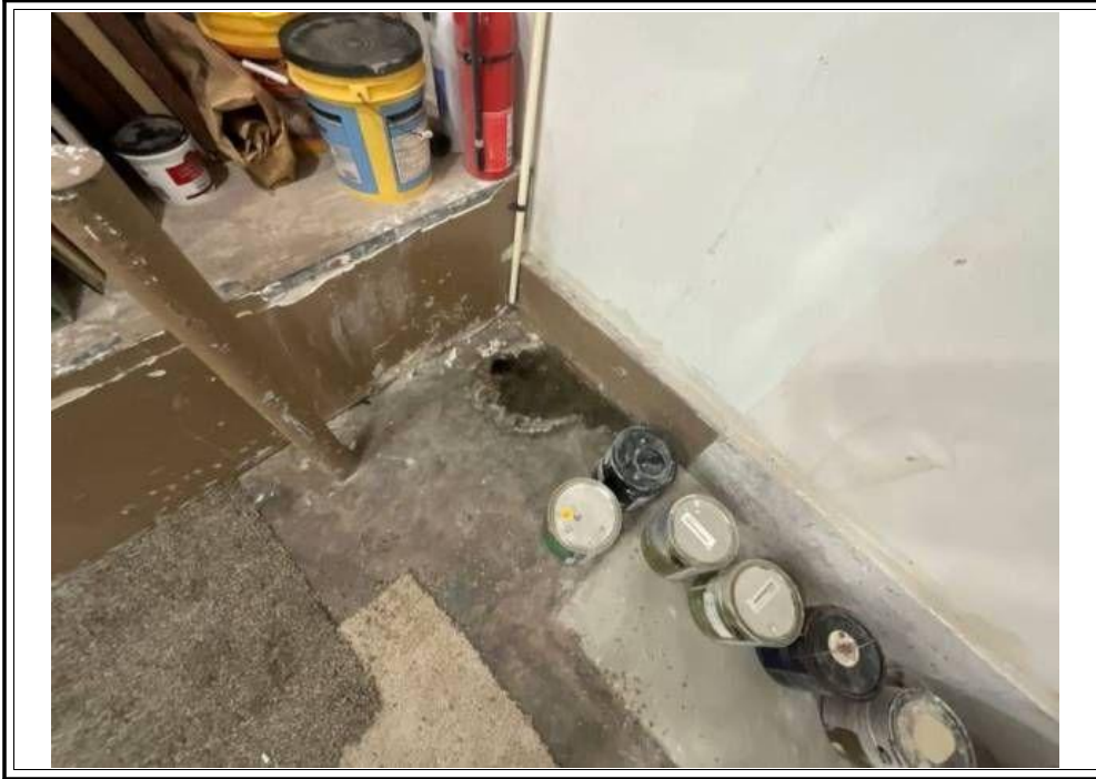
EVIDENCE OF DAMPNES
