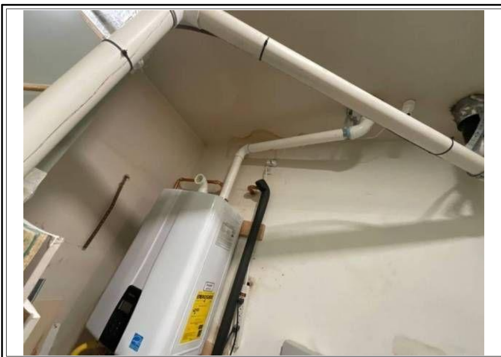
TANKLESS HOT WATER HEATER EVIDENCE OF DAMPNES
