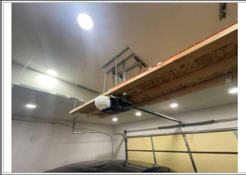
GARAGE AUTOMATIC GARAGE DOOR OPENER
