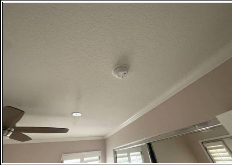
BEDROOM 3 SMOKE DETECTOR
