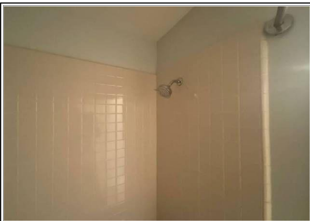
BATHROOM 2 BATHROOM SHOWER HEAD
