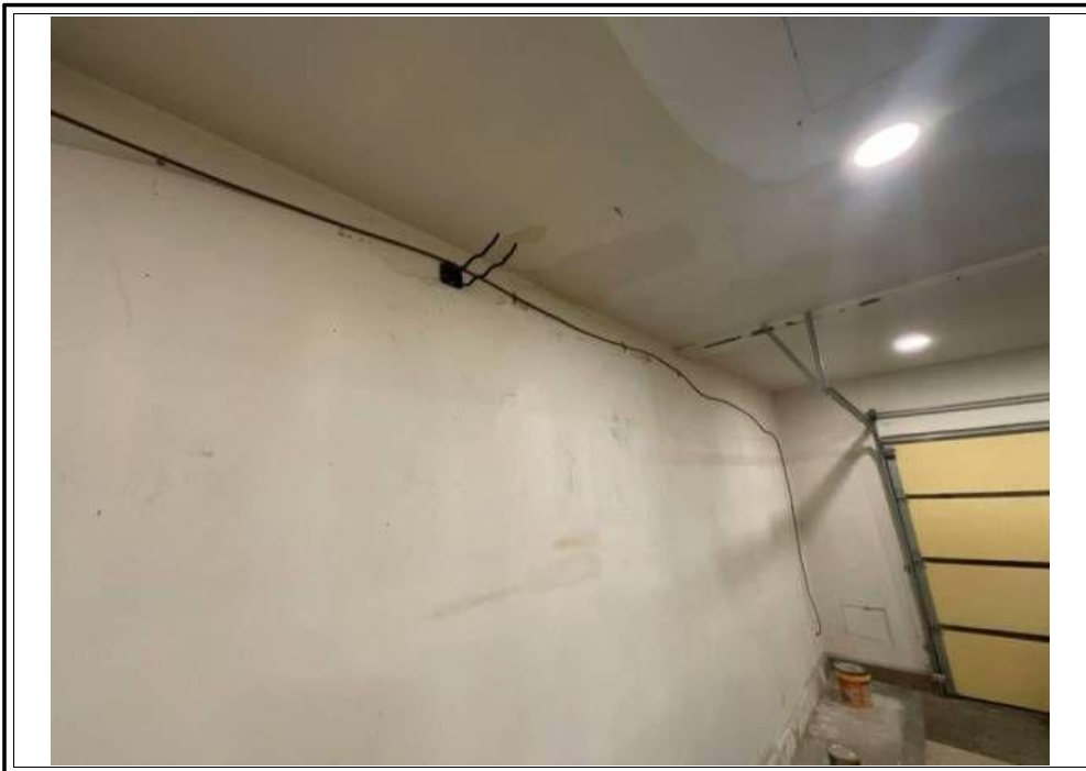
GARAGE EVIDENCE OF DAMPNES
