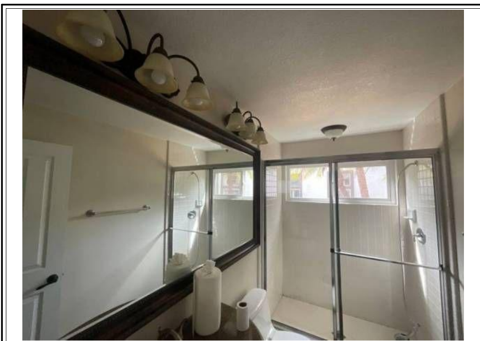
BATHROOM 1 TRACK LIGHTING
