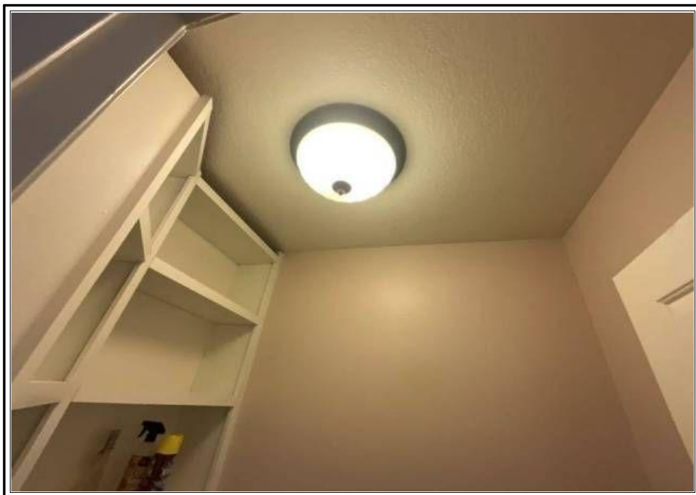
BATHROOM 3 LIGHT FIXTURES
