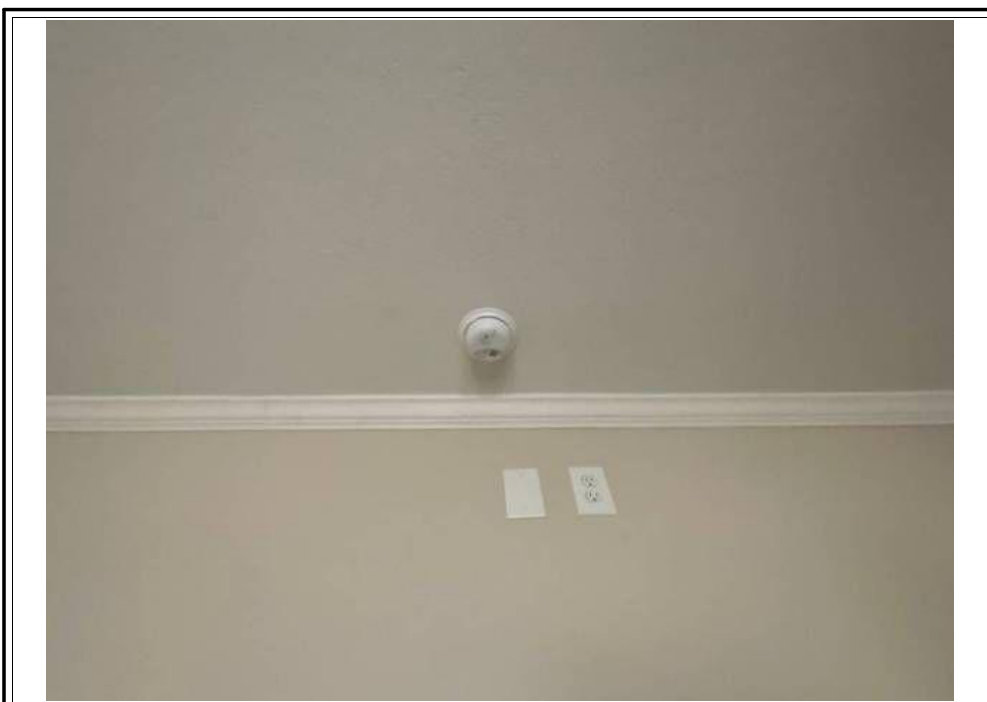
BEDROOM 1 SMOKE DETECTOR
