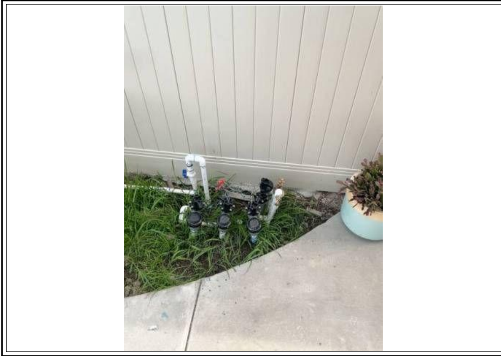
AUTOMATIC SPRINKLER SYSTEM
