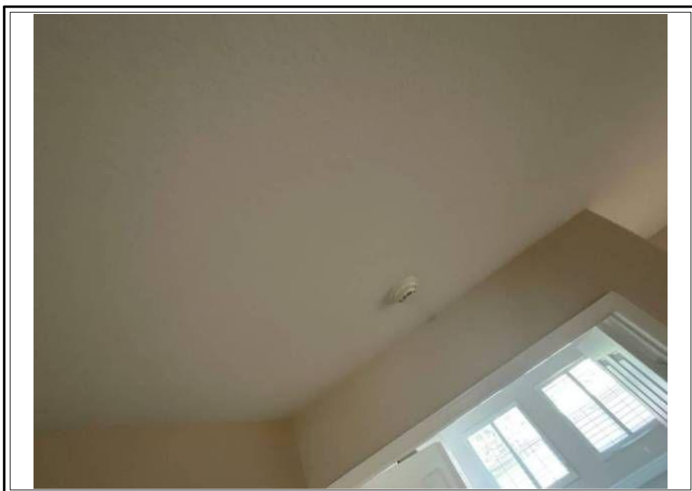
SMOKE DETECTOR CARBON MONOXIDE MONITOR
