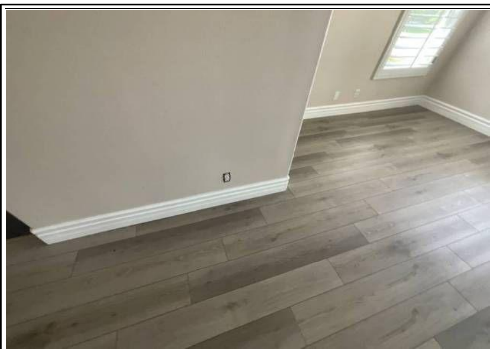
BEDROOM 4 MISSING COVER OUTLET
