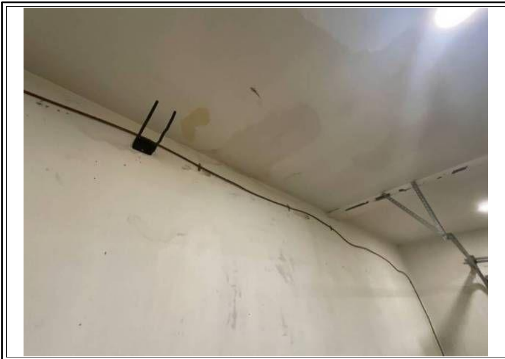
EVIDENCE OF DAMPNES
