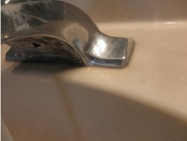
Leak at the left sink faucet in the master bathroom.
