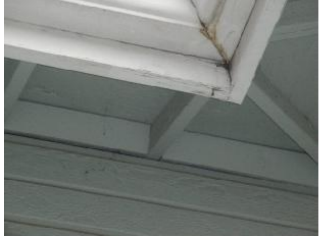
Moisture damage at the fascia board.
