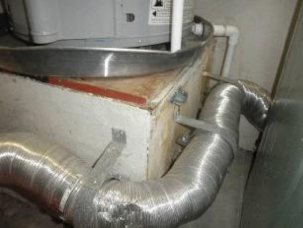
Minor moisture damage to the water heater platform.
