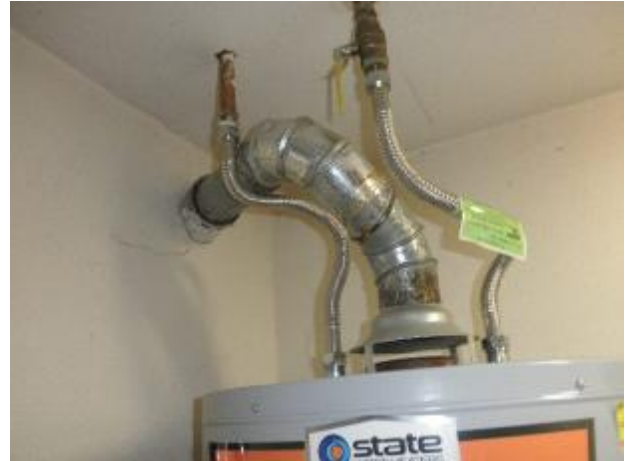
Screws missing at the water heater exhaust.
