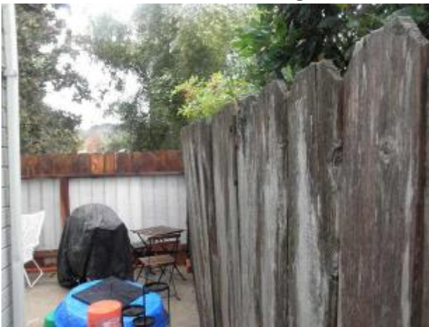
Part of the fence in the backyard is leaning.
