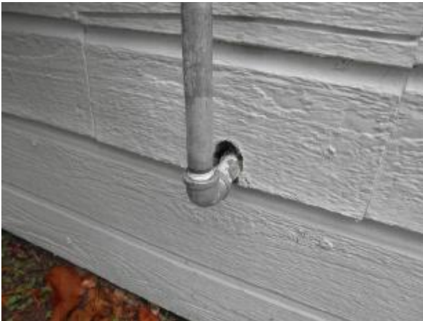
Seal the gap where the gas line penetrates the exterior wall.
