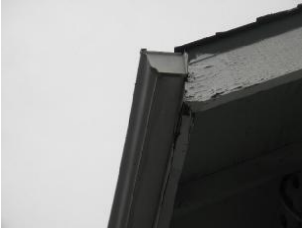
Moisture damage at the fascia board.
