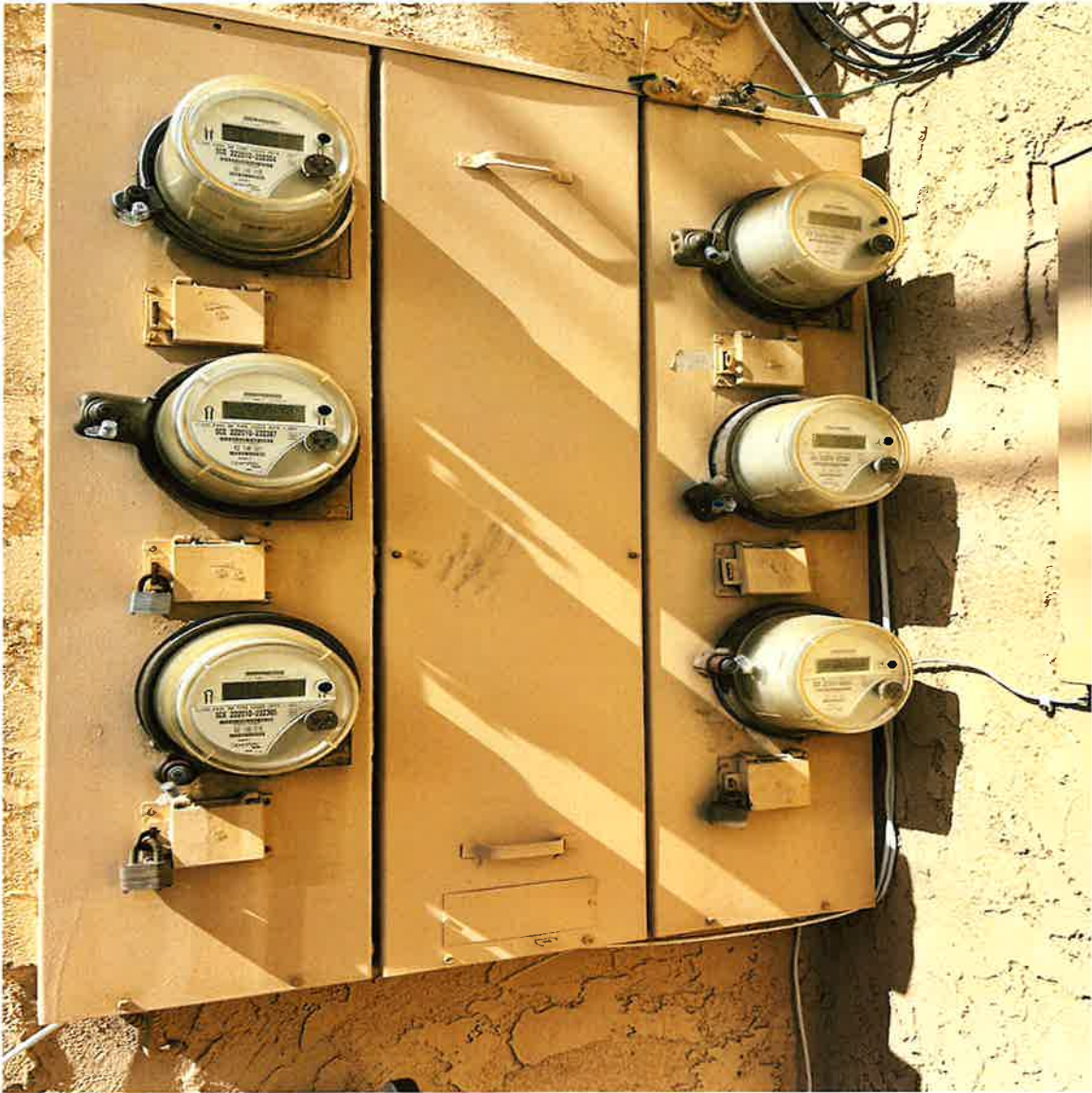
The property features separately metered electricity for each unit.
