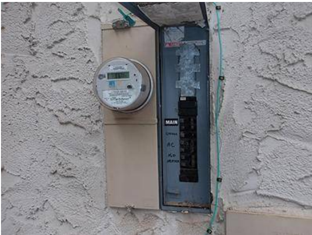
Photo 47-1 Meter & main panel
