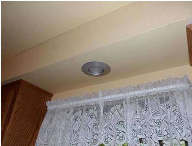
Photo 16-2 Kitchen sink light
