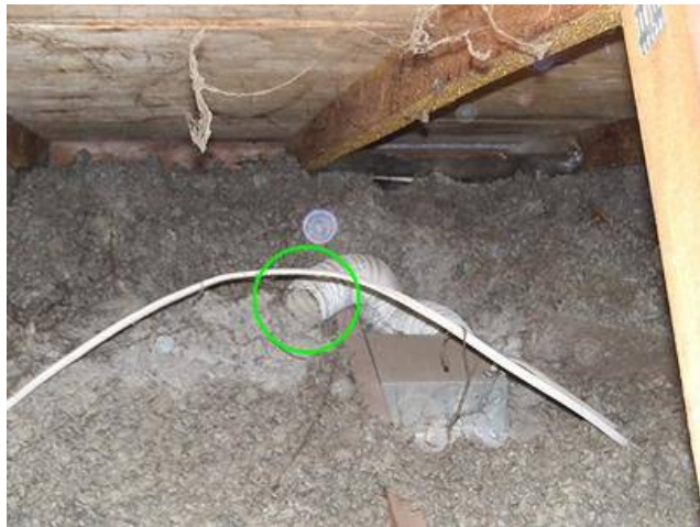
Photo 19-2 Master bathroom exhaust fan & duct
