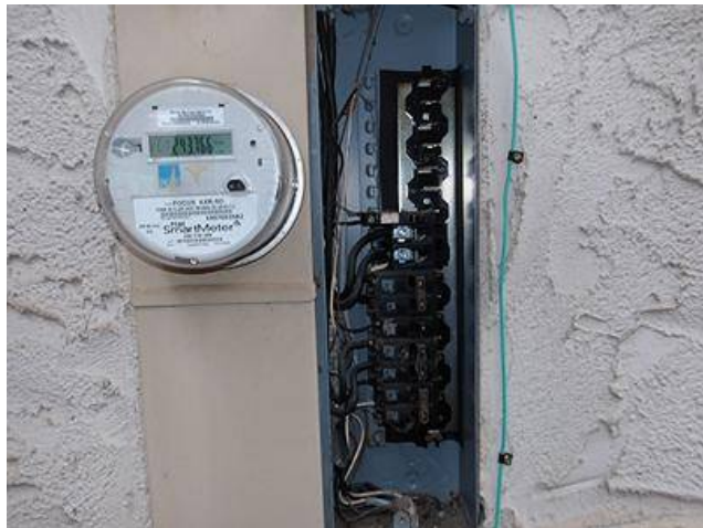
Photo 47-2 Meter & main panel
