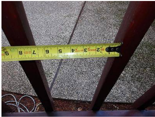
Photo 2-2 Front porch guardrail
