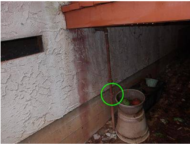
Photo 52-1 Gas shut-off valve, West side
