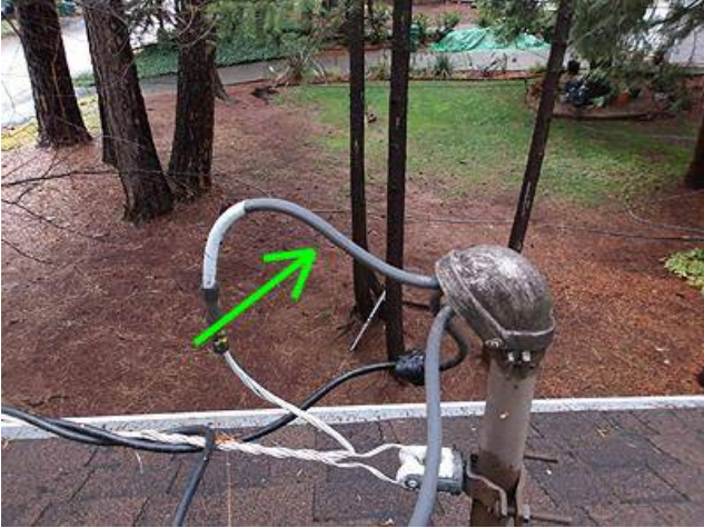
Photo 37-1 Electric service mast
