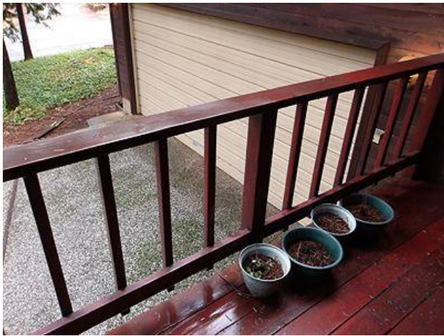
Photo 2-1 Front porch guardrail
