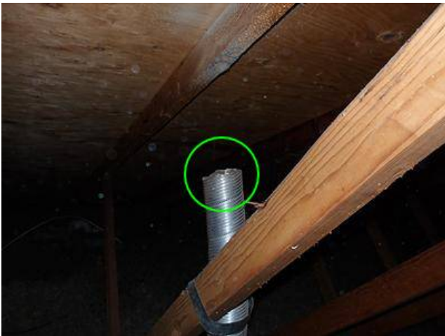
Photo 19-1 Hall bathroom exhaust fan duct
