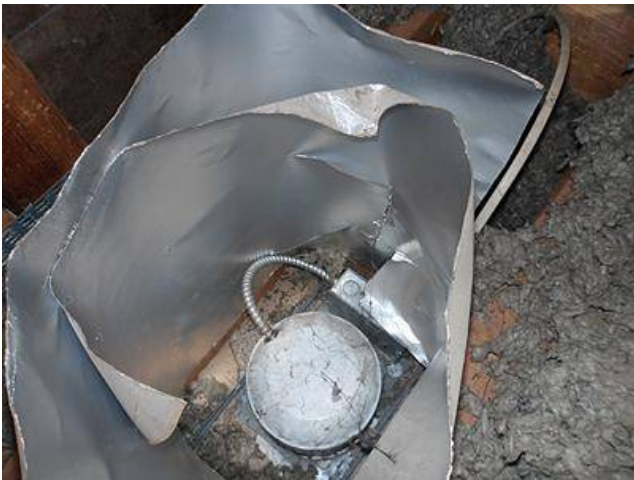
Photo 16-1 Kitchen sink light
