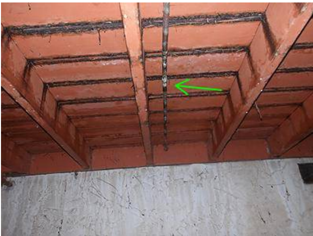
Photo 49-1 Water line below West deck
