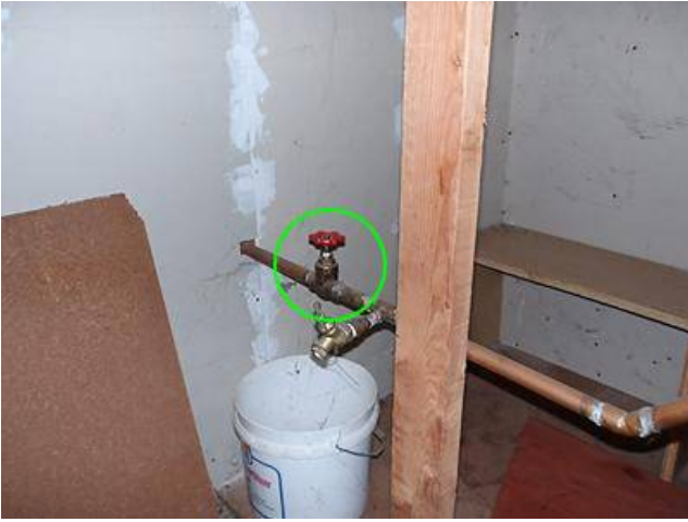
Photo 49-3 Shut-off valve for West deck hose bib
