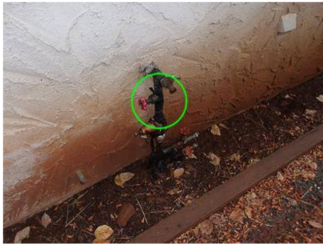
Photo 52-2 Water shut-off, SW corner garage
