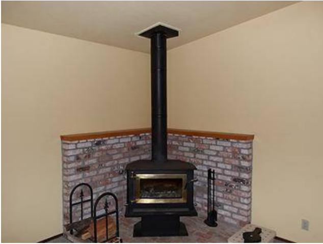
Photo 58-1 Wood stove & chimney
