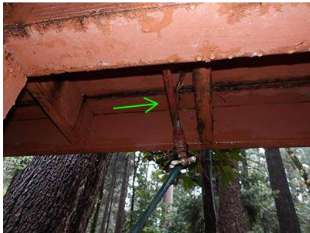
Photo 49-2 Hose bib below West deck
