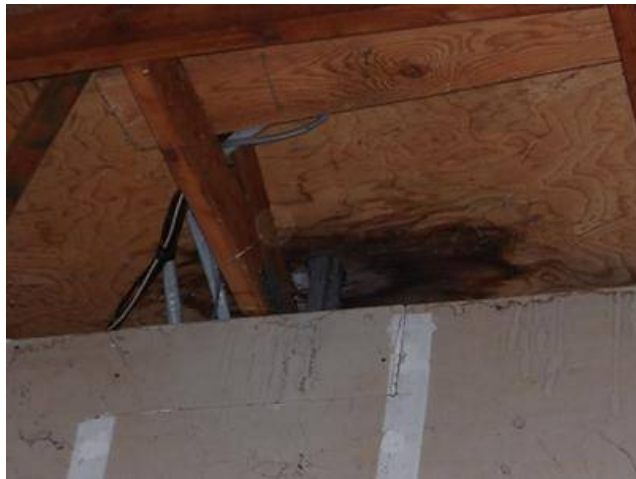
Photo 27-2 In garage at electric service mast penetration
