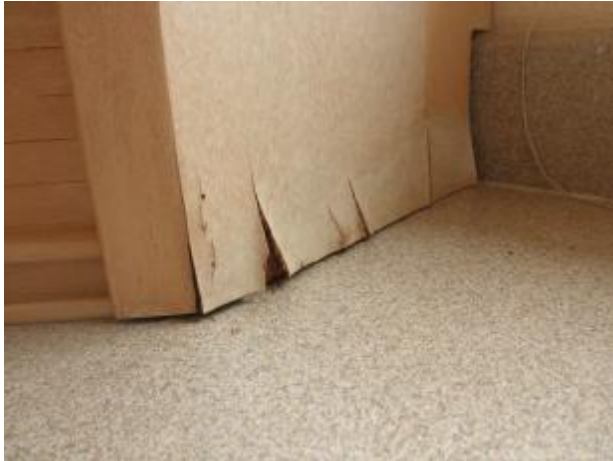
Moisture damage to the side of the cabinet.
