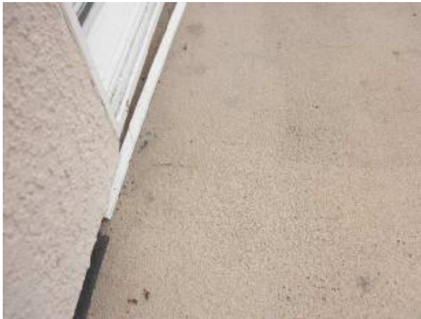
Surface cracking at the deck water proof coating.
