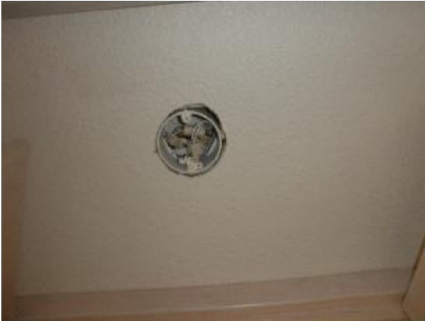
Junction box missing cover plate in the laundry area.
