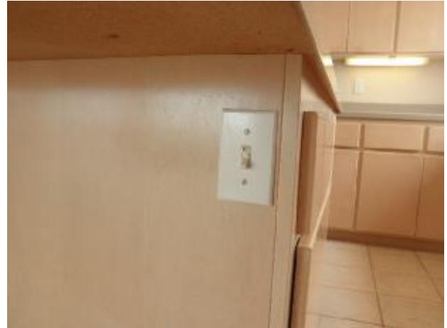
Garbage disposal switch at the side of the island.
