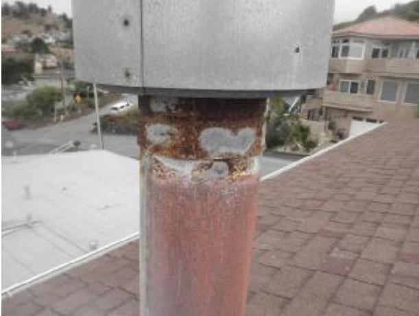
Rust damage at the chimney exhaust.
