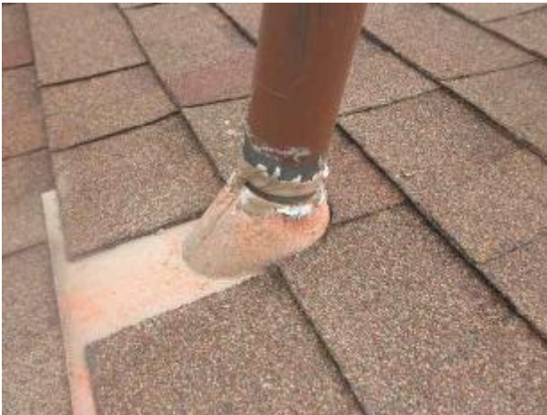
The flashings need to be resealed.
