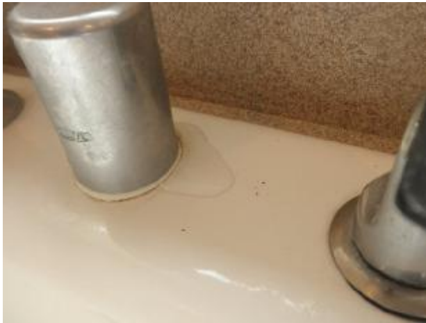
Water drains out of the air gap.
