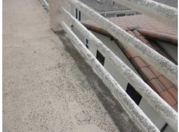
General deterioration of the deck coating due to age.
