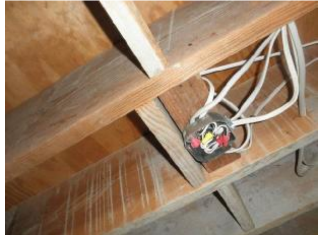
Example of open junction boxes in the shop.
