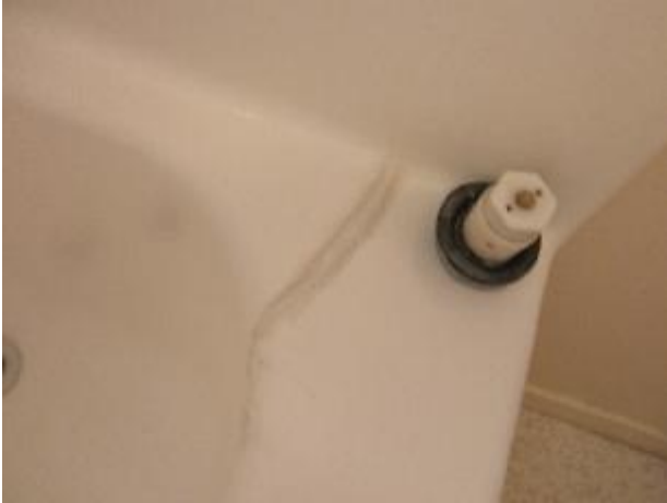
Sealed crack at the hall bathroom tub.
