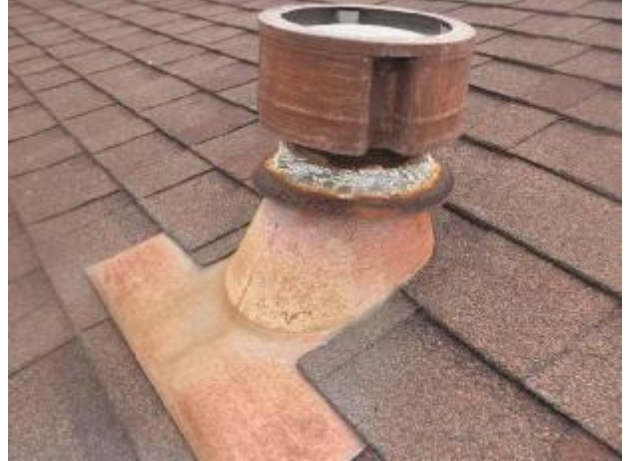
Rust damage at the furnace exhaust.
