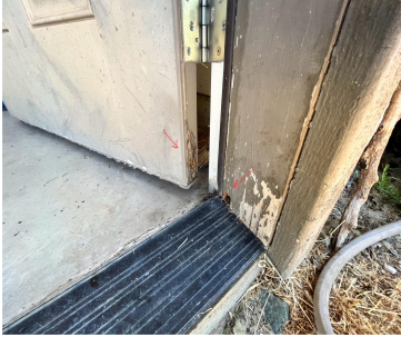
3D - Damage to pedestrian garage door
