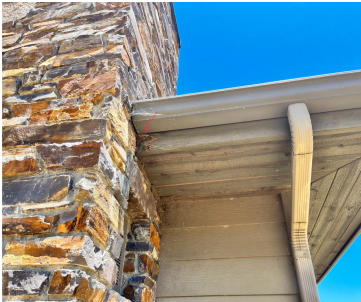
3A - Damage to the fascia board
