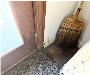
3E - Damage to baseboards
