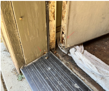
3C - Damage to laundry room door
