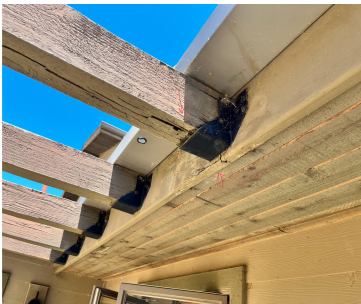
3A & 3B Example of damage to the fascia and patio framing.
