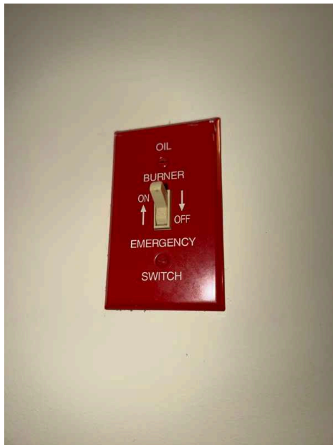
Emergency shut off located at the bottom of the basement stairs
