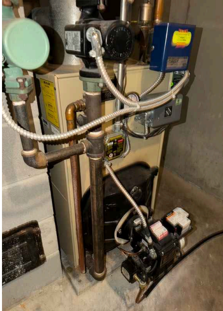
Boiler operational at time of inspection.
