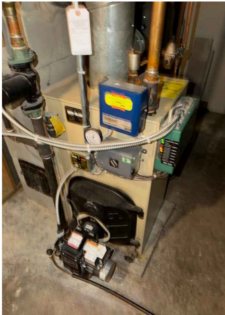
Boiler operational at time of inspection.
