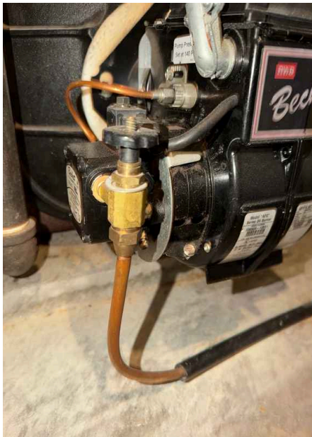
Located at boiler
