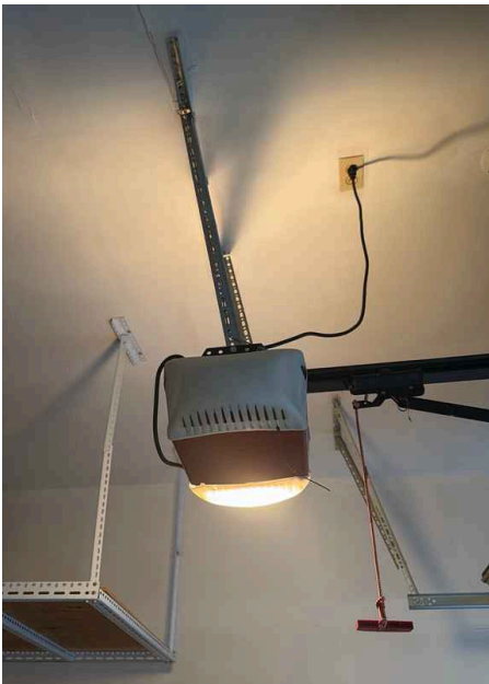
Garage door opener operational at time of inspection.
