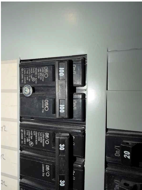
Home provide provided with 100 amp service.
