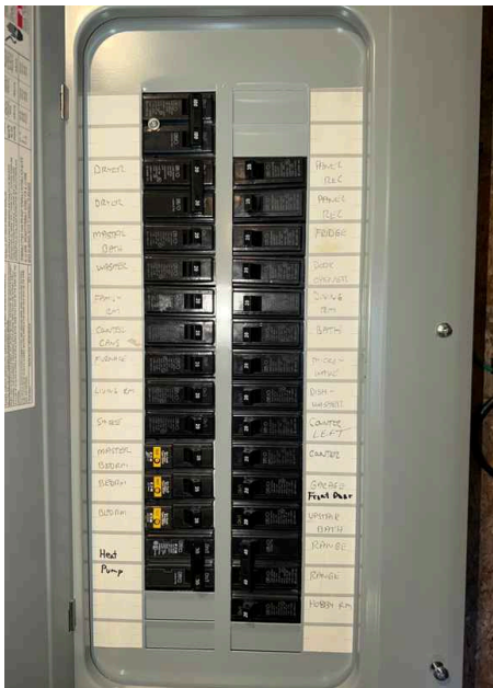
Main panel inspected by the boiler with no major concerns observed.
