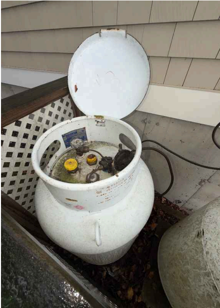
Propane tank found to be in good condition.
