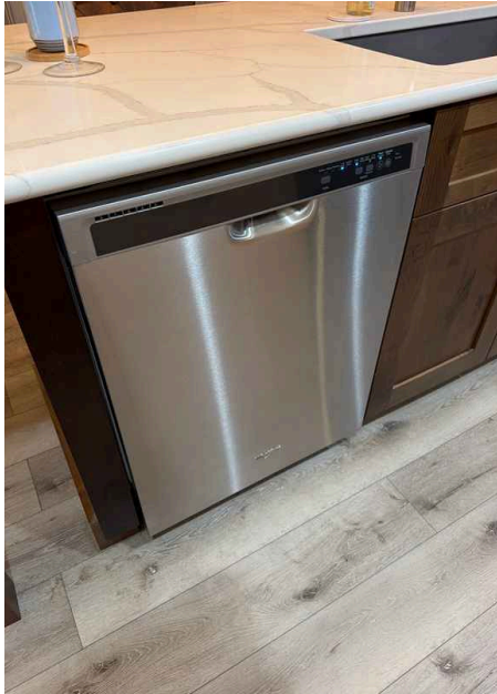
Dishwasher operational at time of inspection.
