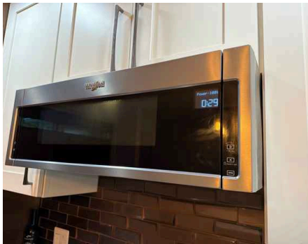
Microwave operational at time of inspection.
