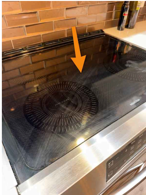
Unable to test operation of the cooktop as it is induction and there was no cookware present at the property during the inspection.
