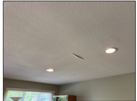
Loose material observed - needs to be serviced
