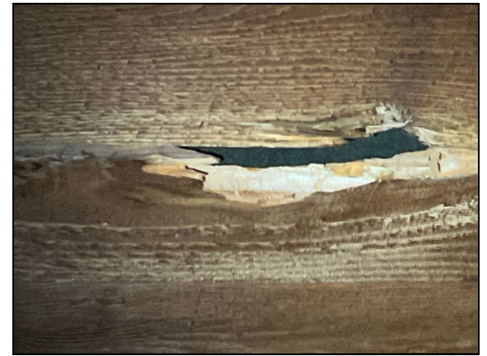
Cracking large- needs to be serviced
