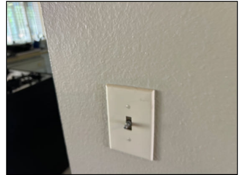
Dimmer switch knob missing
