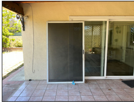
Off tracks - needs to be serviced
