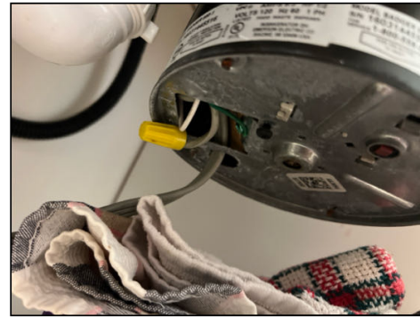
Exposed wire connections - needs to be serviced
