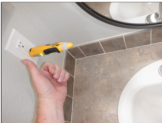
5.8 Item 1(Picture) Good GFCI
