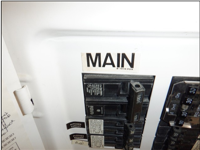
8.0 Item 3(Picture) Main 100 amp breaker
