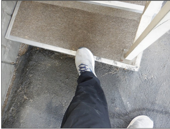
2.3 Item 2(Picture) Loose trim on steps
