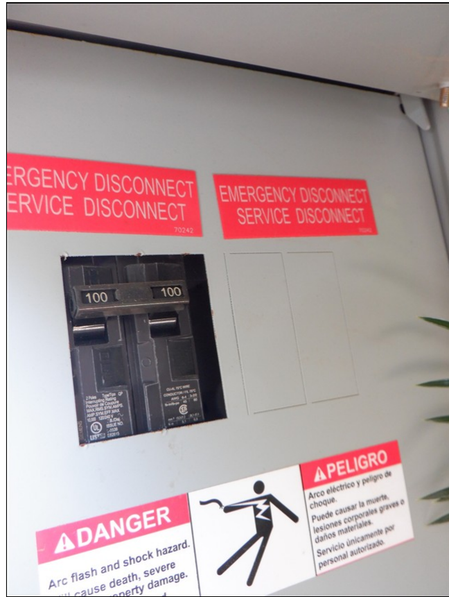
8.4 Item 2(Picture) Main 100 amp breaker
