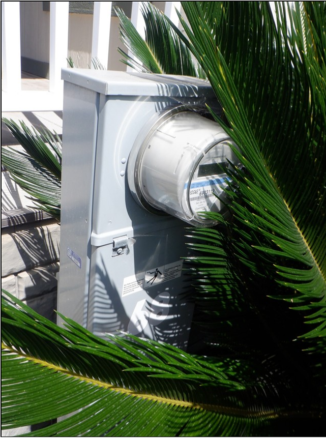
8.4 Item 1(Picture) Electric meter
