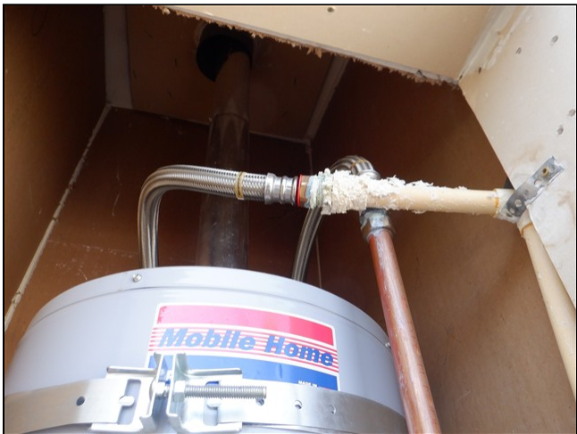
7.1 Item 5(Picture) Corrosion
