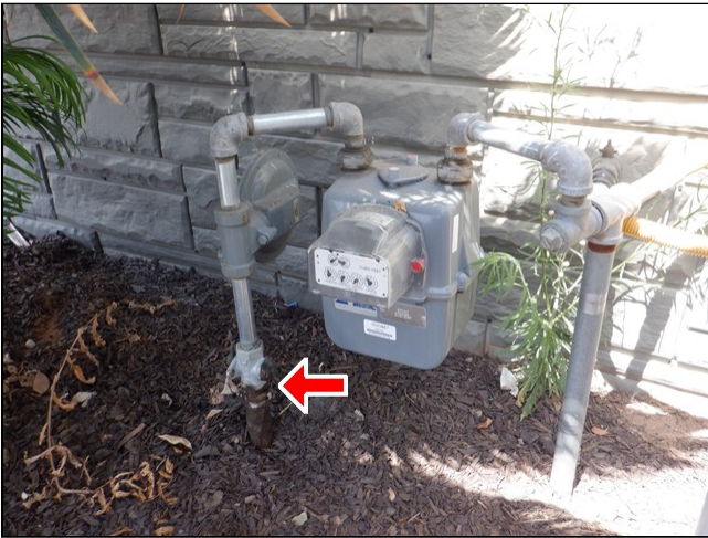
7.4 Item 1(Picture) Gas meter and shut off
