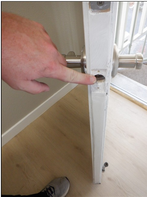
2.1 Item 1(Picture) Missing latch on laundry room exterior door
