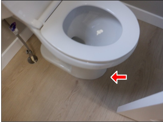
5.7 Item 6(Picture) Loose primary bath toilet
