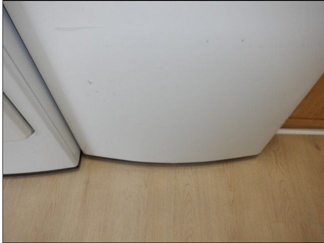
3.13 Item 2(Picture) Missing drip pan under washer
