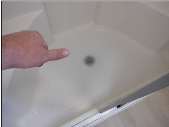
5.6 Item 2(Picture) Primary bath shower drained slowly
