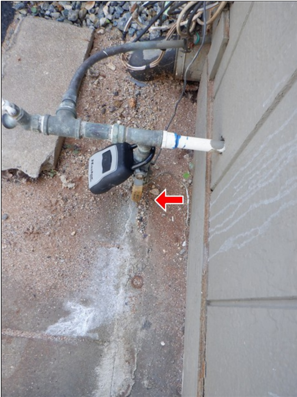
7.2 Item 1(Picture) Main water shut off
