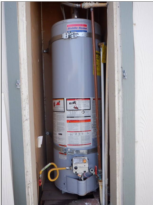
7.1 Item 1(Picture) Water heater
