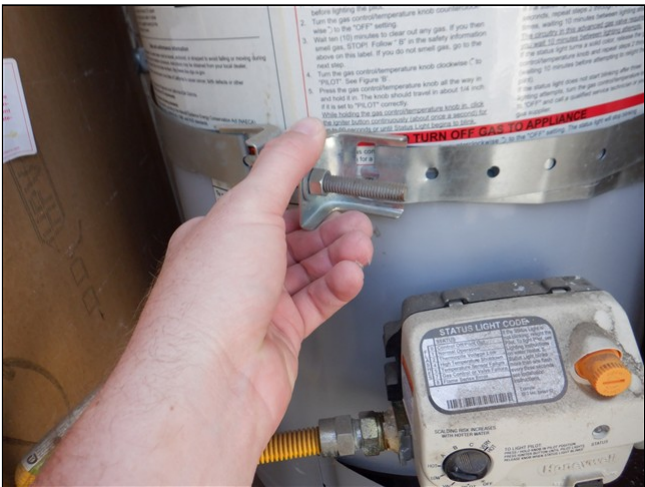
7.1 Item 6(Picture) Loose belly strap
