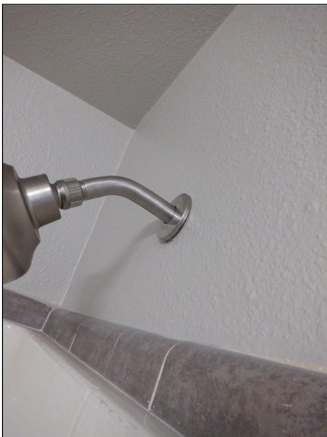
5.7 Item 3(Picture) Hallway bath showerhead not sealed
