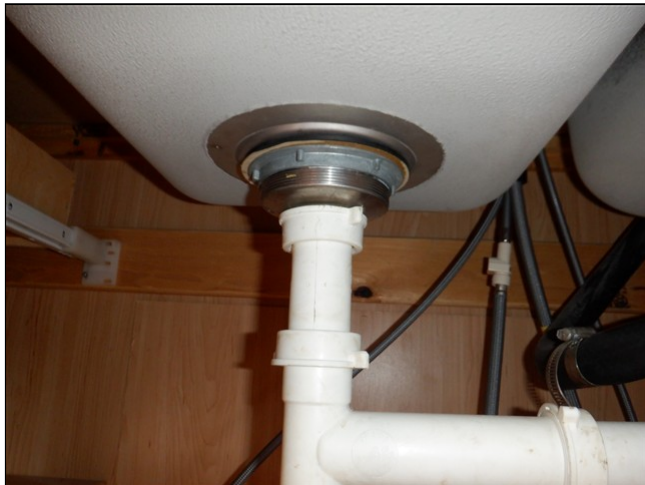
3.5 Item 2(Picture) Kitchen sink plumbing / no leaks
