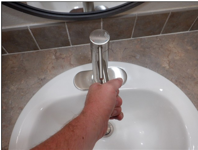
5.7 Item 1(Picture) Loose faucet in hallway bath
