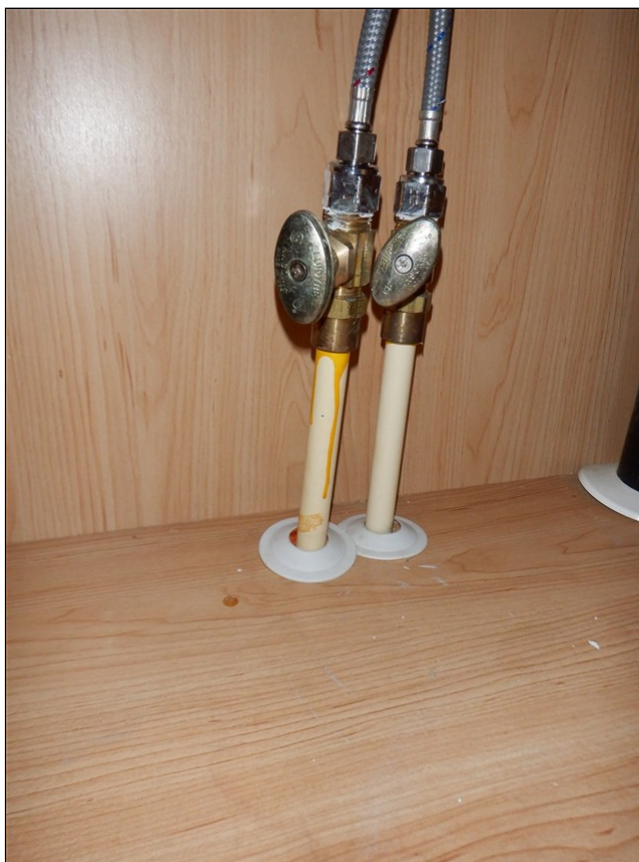
5.7 Item 4(Picture) CPVC plumbing
