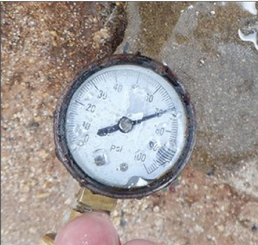
2.6 Item 1(Picture) Water pressure
