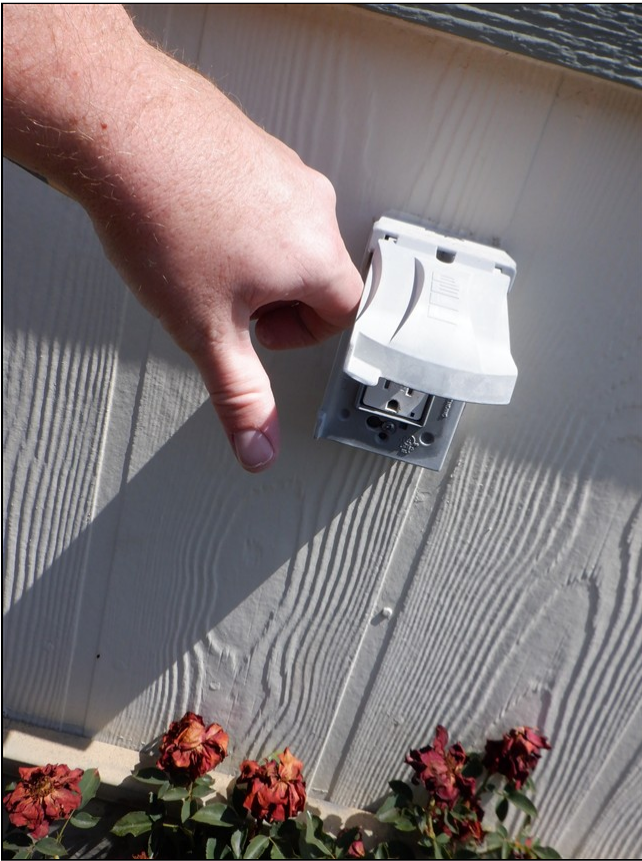
2.7 Item 1(Picture) Bad GFCI on left side of home
