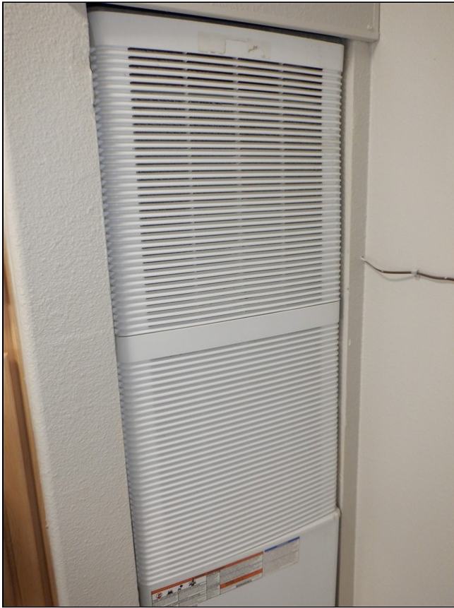
9.0 Item 1(Picture) Furnace
