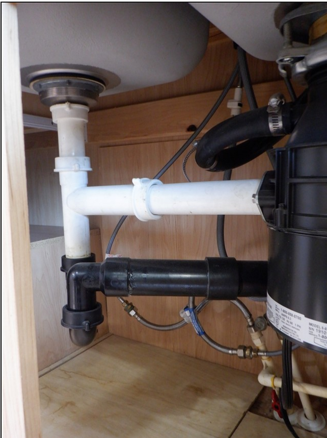
3.5 Item 1(Picture) Kitchen sink plumbing / no leaks
