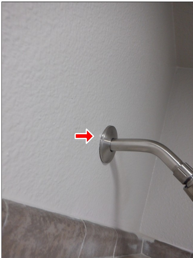
5.7 Item 8(Picture) Primary bath showerhead not sealed
