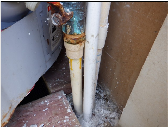
7.1 Item 4(Picture) Corrosion
