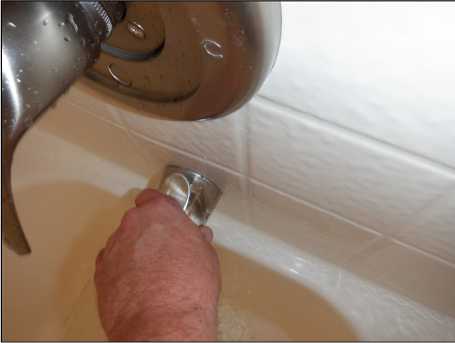
5.7 Item 5(Picture) Tub faucet not sealed
