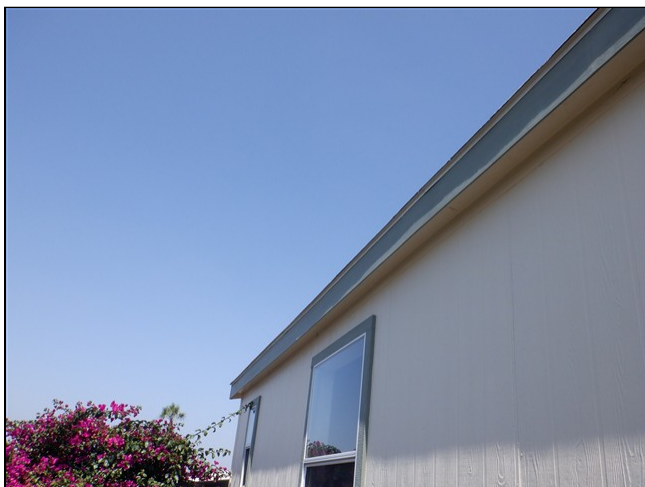
1.2 Item 1(Picture) No gutters
