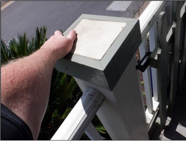
2.3 Item 1(Picture) Loose railing on front porch
