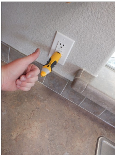
3.7 Item 1(Picture) Good GFCI
