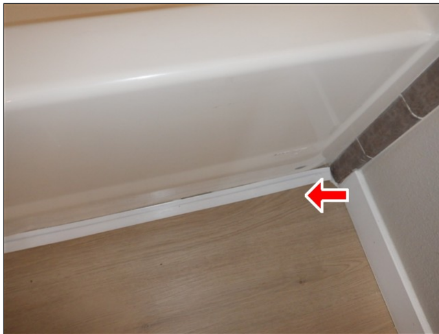
5.7 Item 2(Picture) Loose trim at base of tub
