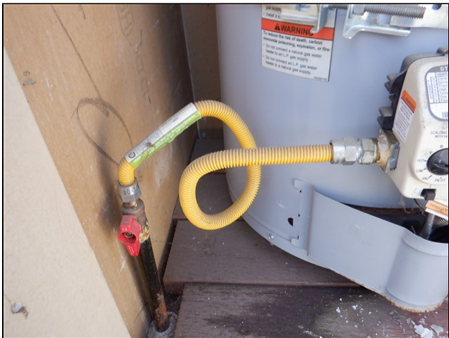
7.1 Item 3(Picture) Missing sediment trap
