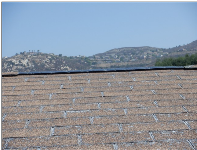
1.0 Item 14(Picture) Missing ridge line shingles
