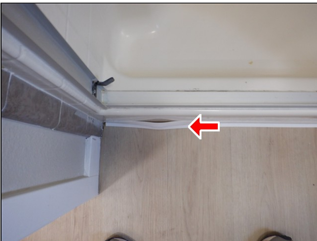
5.7 Item 7(Picture) Loose plastic stripping on primary bath shower
