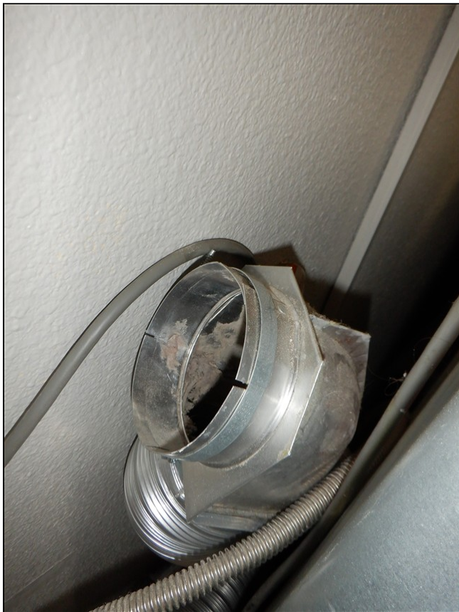
3.13 Item 5(Picture) Dryer vent not connected
