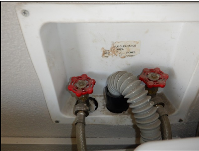
3.13 Item 3(Picture) Washer valves / drain
