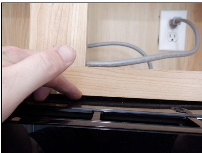
3.10 Item 1(Picture) Fan venting under cabinet
