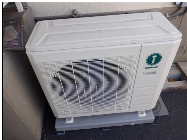
9.5 Item 1(Picture) Condenser
