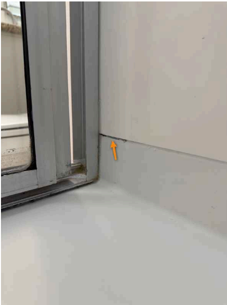
Example Noted at Master Bathroom
