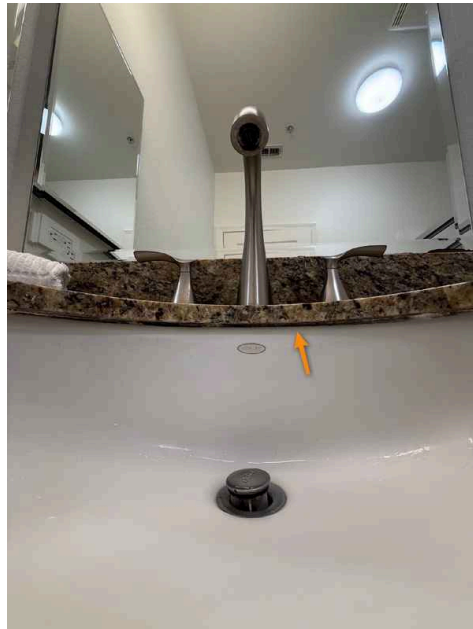
Example Noted at Master Bathroom
