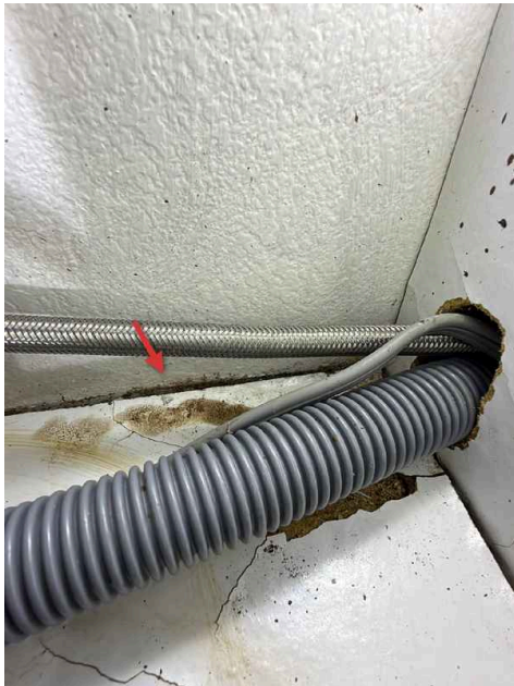
Example Noted Below the Kitchen Sink
