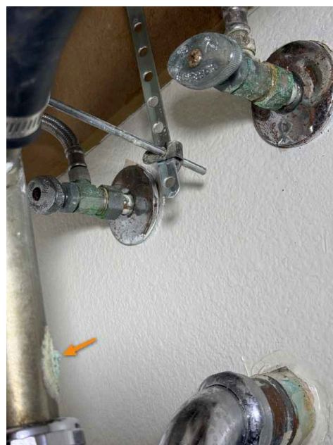
Example Noted at Hall Bathroom
