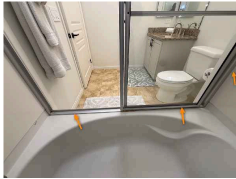
Example Noted at Master Bathroom
