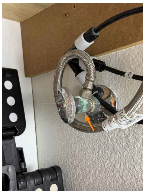
Example Noted at Master Bathroom
