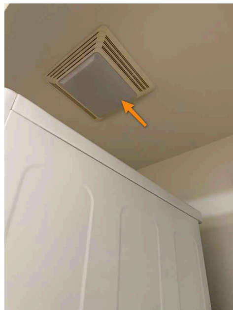
Example Noted at Laundry Room
