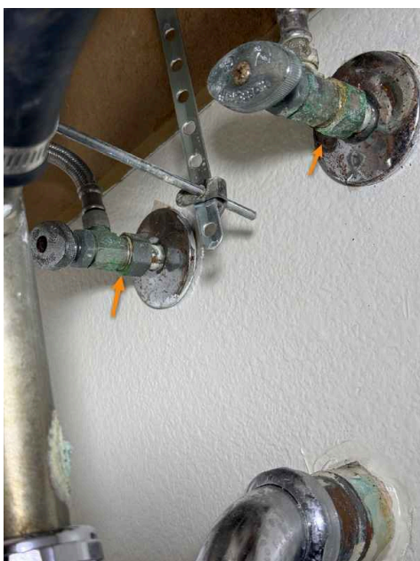
Example Noted at Hall Bathroom
