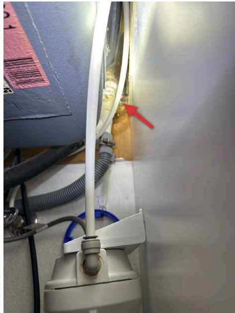
Example Noted at the underside of the Kitchen Counter top (Near the AirGap)
